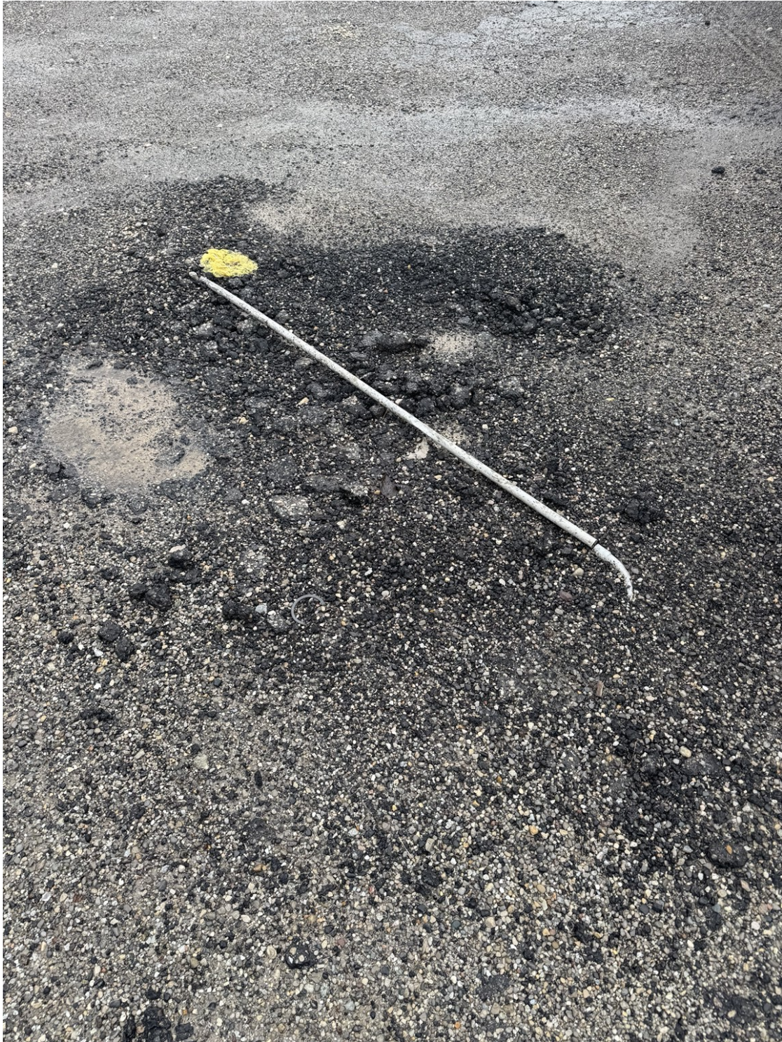
Figure A2. Close view of failed asphalt / patching and deteriorated surface conditions.
