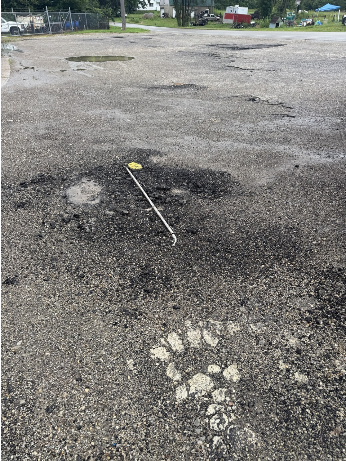
Figure A3. Wider front-area view showing potholes, patching, uneven pavement, and ponding across the base-bid work area.
