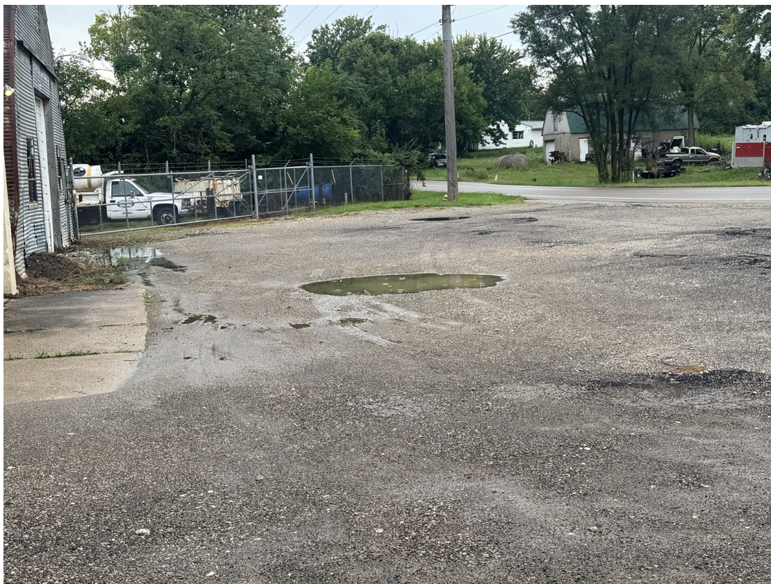
Figure A1. Overall front paved area showing widespread deterioration, standing water / ponding, and failed pavement conditions.
