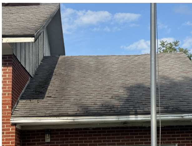
Figure 6. Lower roof slope with visible weathering and valley conditions.
