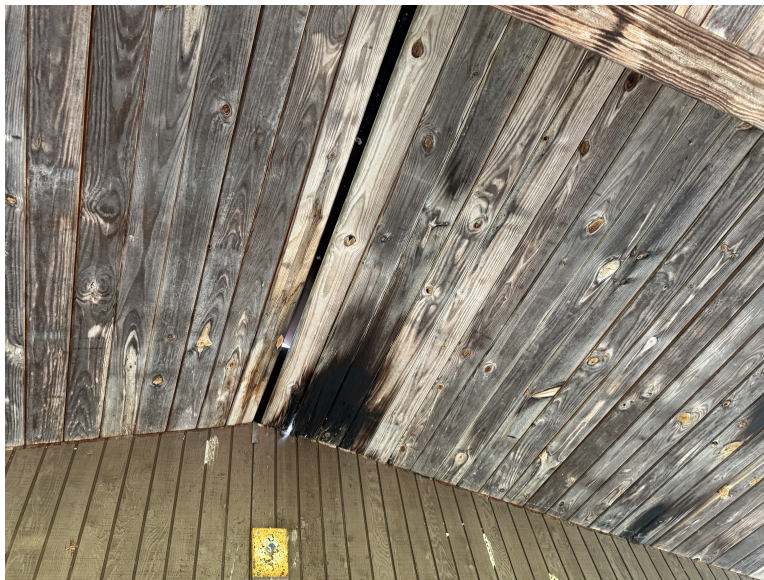
Figure 2. Interior wood ceiling / roof deck condition showing open jointing and visible gaps between boards at the shelter underside.
