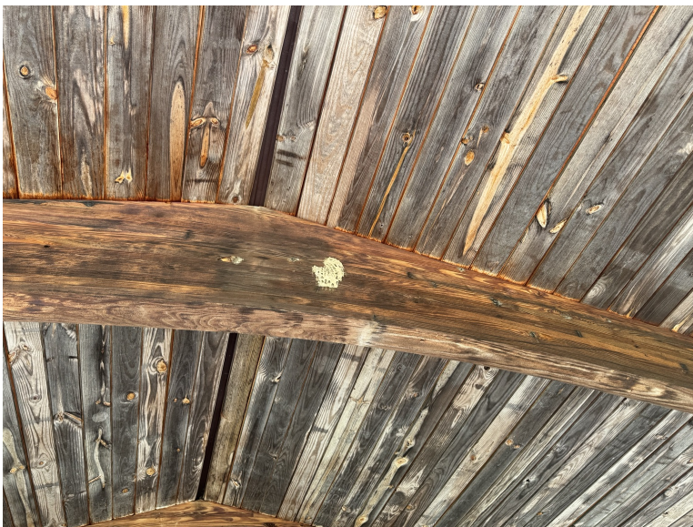
Figure 3. Exposed underside framing and wood ceiling / roof decking at the shelter, showing weathering and areas requiring contractor field verification.
