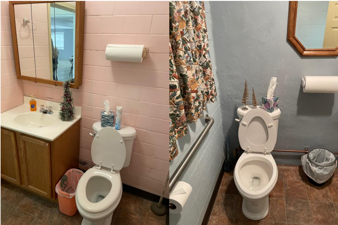
The first photo shows the waiting area for the restrooms with the worn and outdated carpet. Remaining photos illustrate the windows, the outdated décor, and the fixtures that are inadequate for persons with disabilities.
