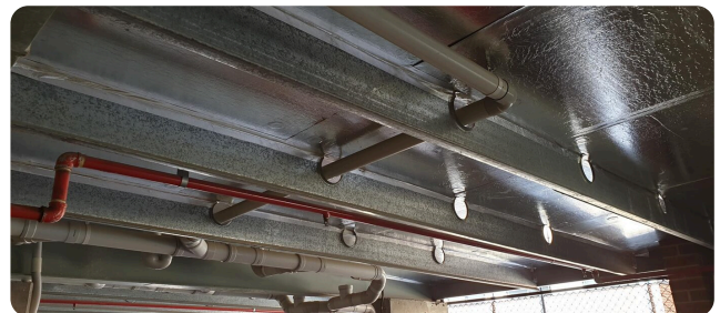
SERVICES THROUGH THE JOIST
