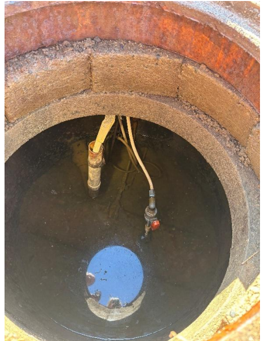
Lancaster Ave chemical injection pit (NaOH & NaOCl) - full of water
