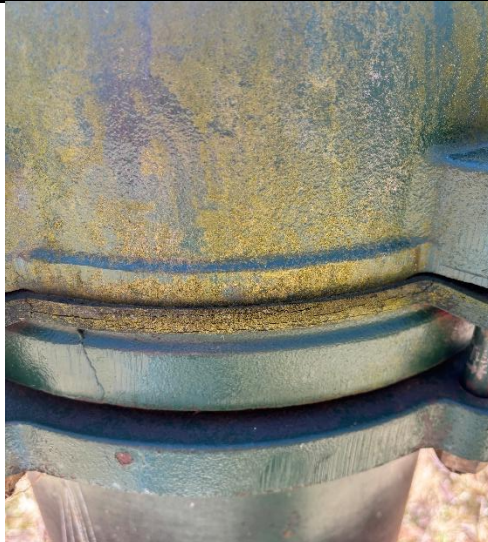
Wellfield 07G: Deteriorating gasket at Well #4
