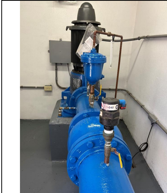
Keating Well (08G) inside pump station
