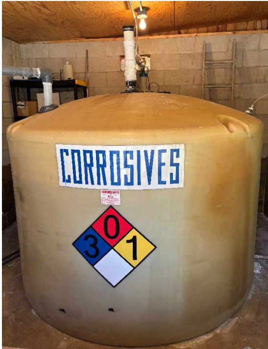
Lancaster Ave Station 1: NaOH bulk tank
