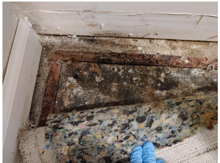
Figure 2-mold under basement carpet
