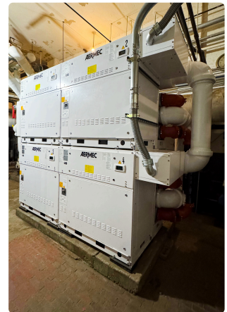
New 120-tons Aermec Modular Chillers
