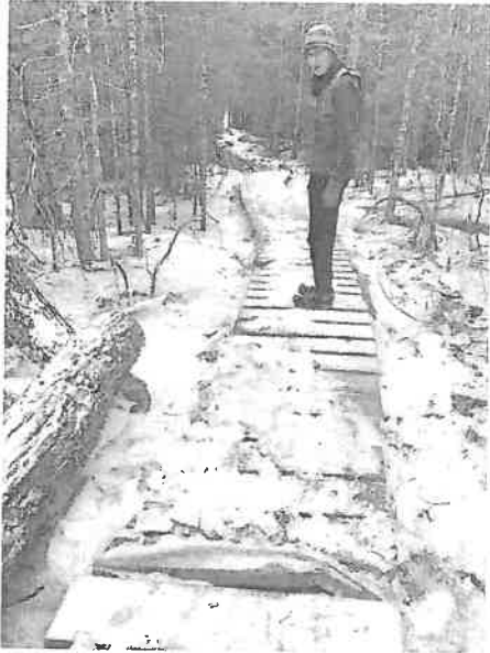
Damage to Half Witt board walk, Norway, Dec 2022
