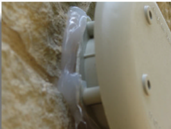
Improper caulk details
