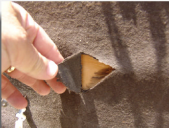
Damages in the moisture barrier
