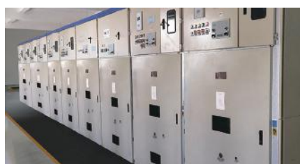
Electricity Distribution Room
