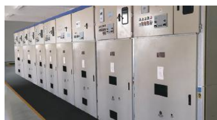
Electricity Distribution Room
