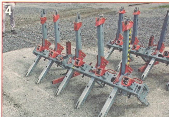
Post impact barrier condition.
