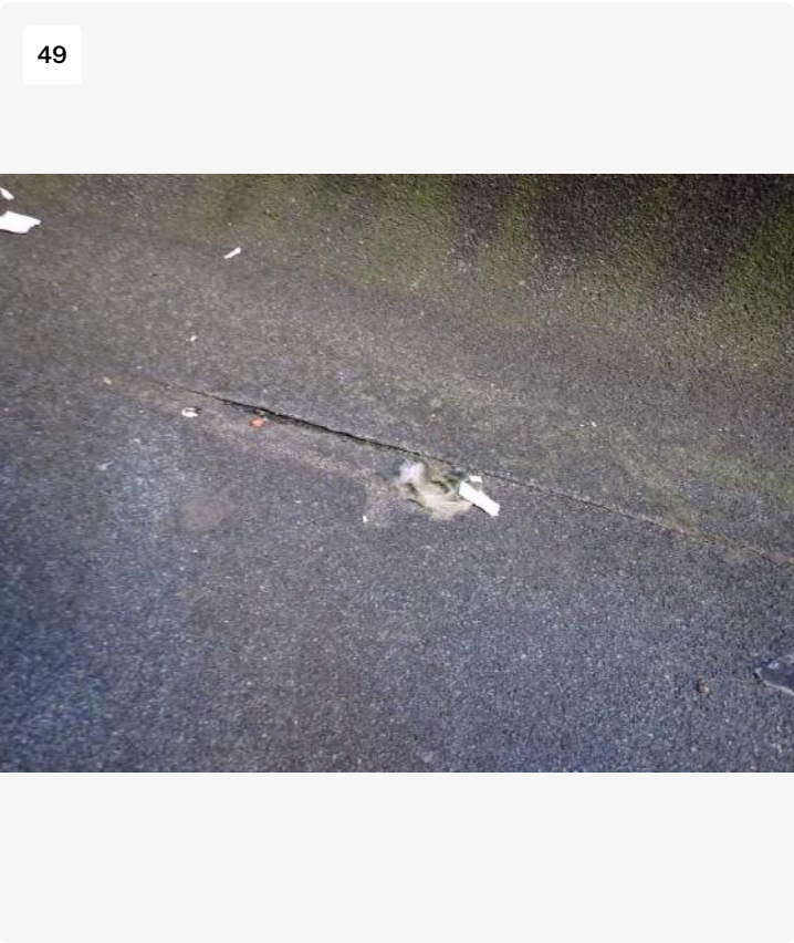
Minor uplift on lap seam
