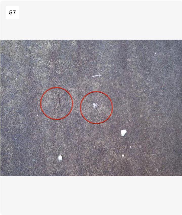
Abrasions in mod-bit from fallen tiles
