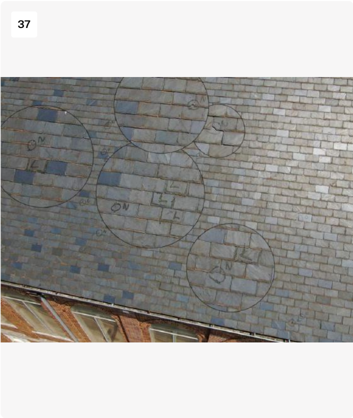
Displaced and broken tiles
