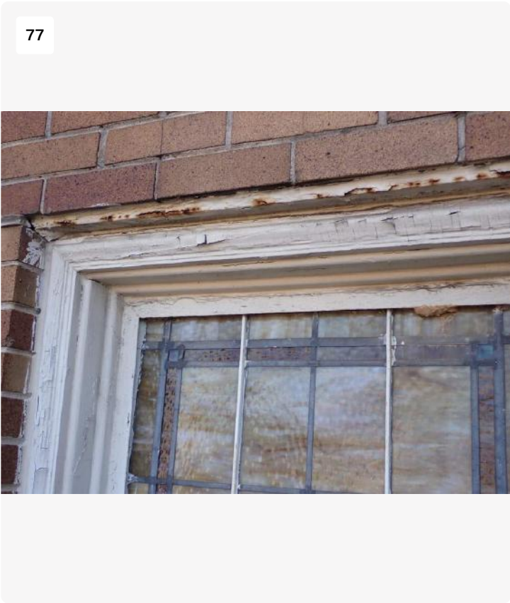
Paint ripped off due to high winds
