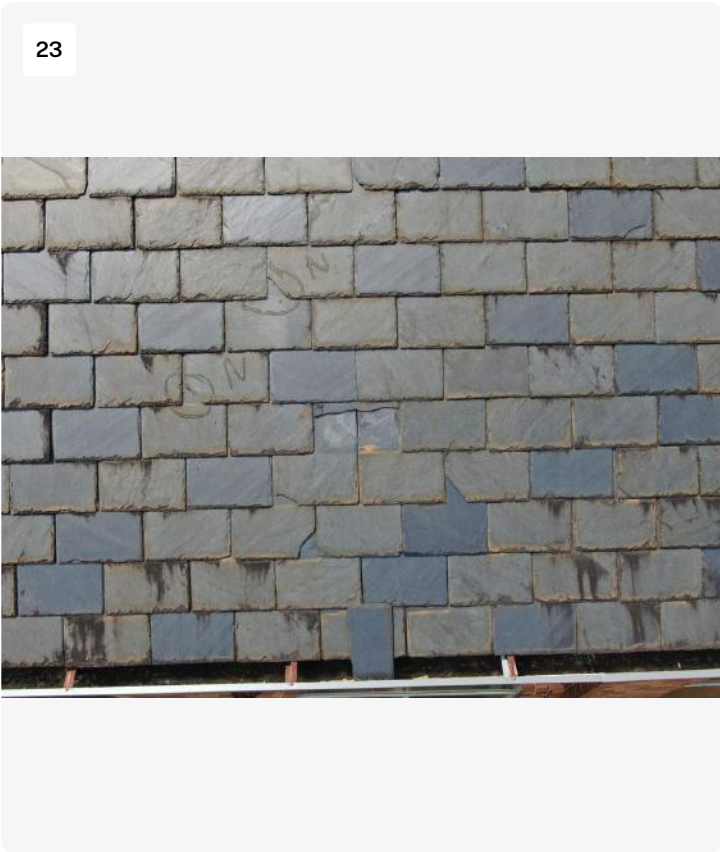
Broken and cracked tiles
