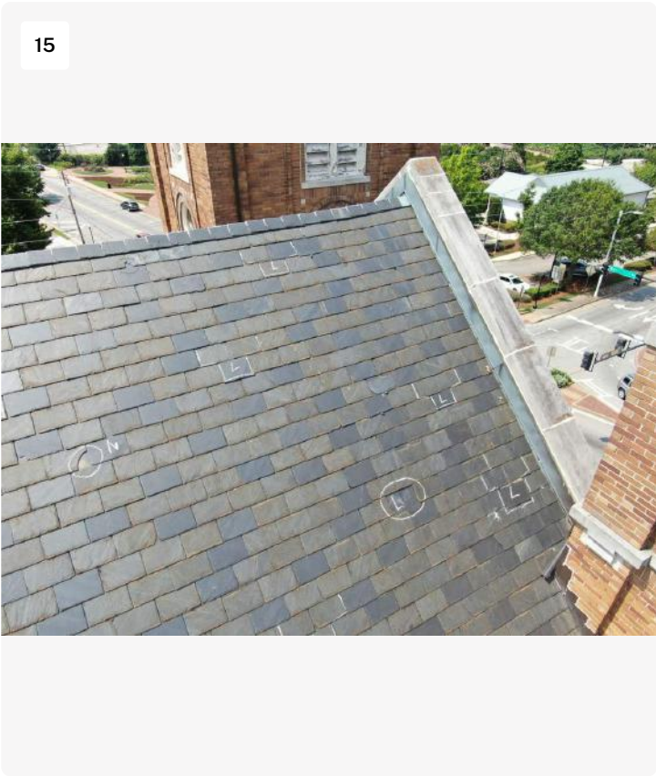
Missing, displaced and chipped tiles noted
