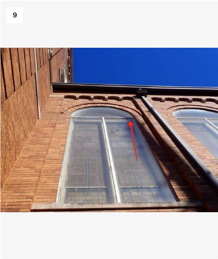
Displaced metal window frame
