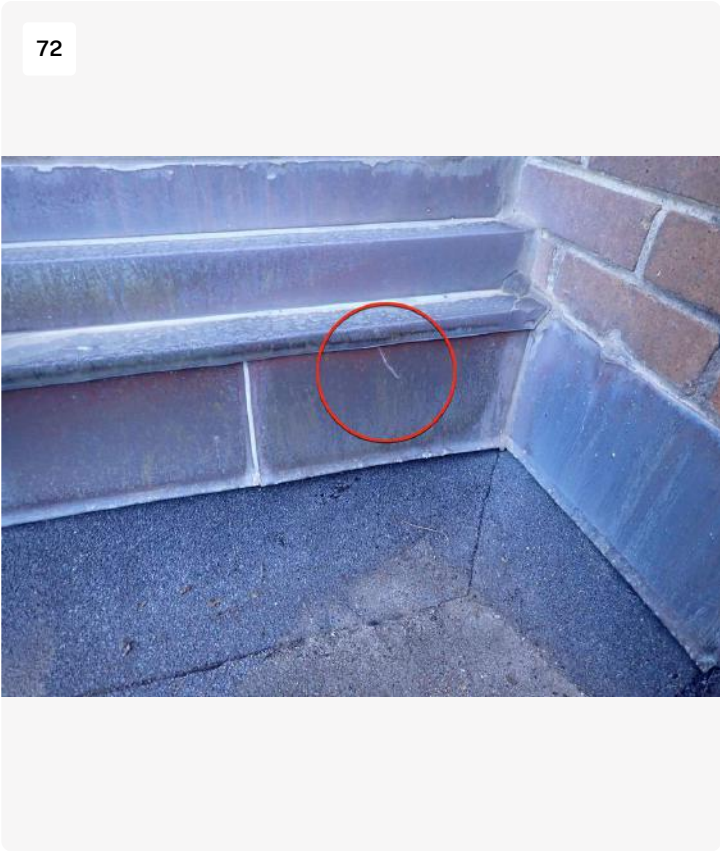
Damage to copper flashing from fallen tile
