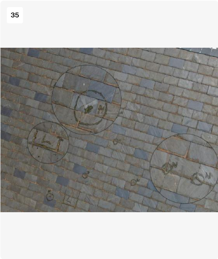
Broken and displaced tiles
