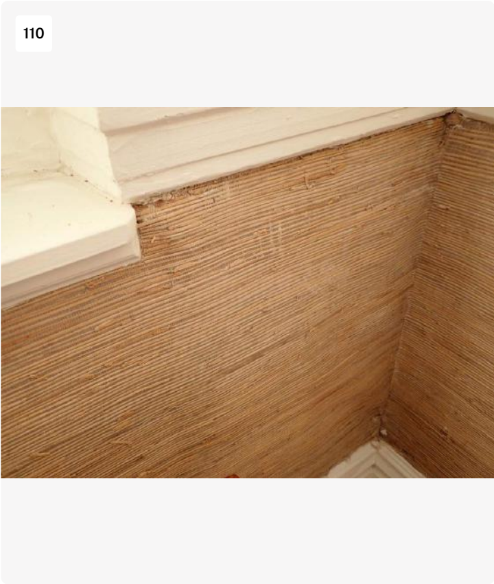
Water intrusion behind wallpaper
