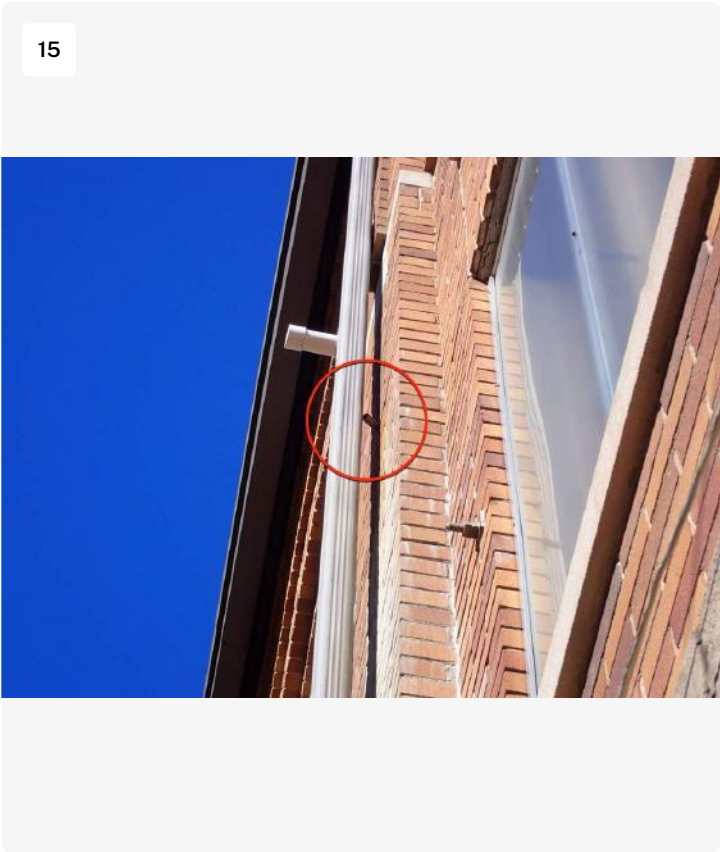
Unknown water line discharge
