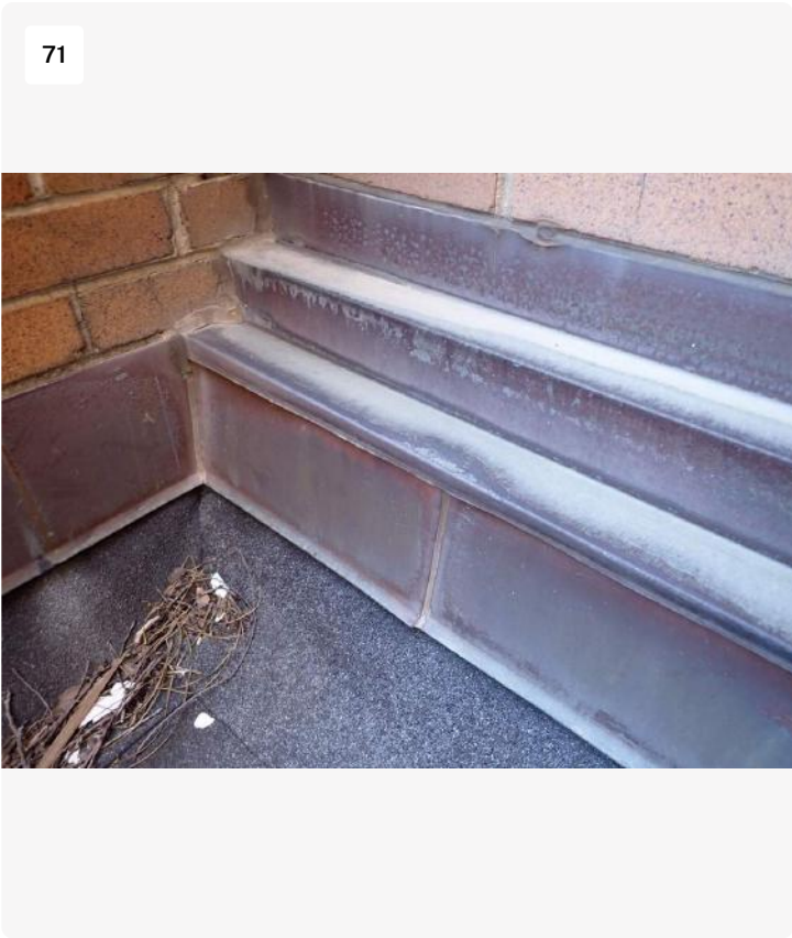
Copper counter flashing
