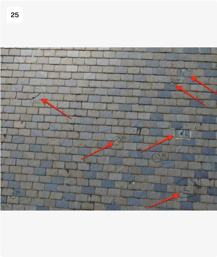
Broken, cracked and displaced tiles
