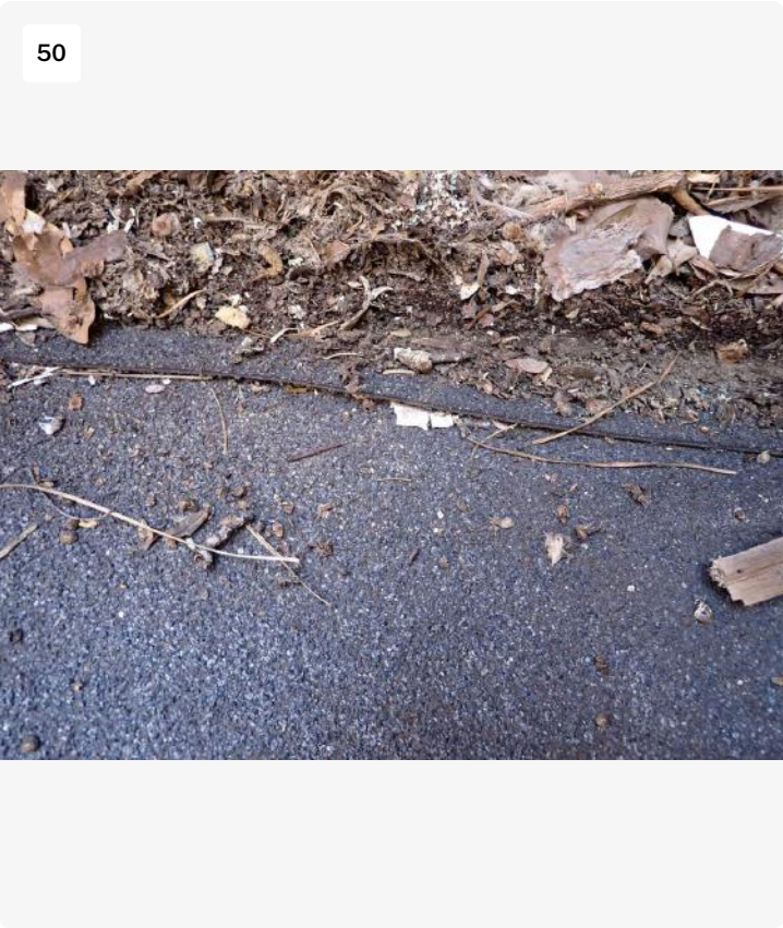
Uplifted lap seam and wind-borne debris
