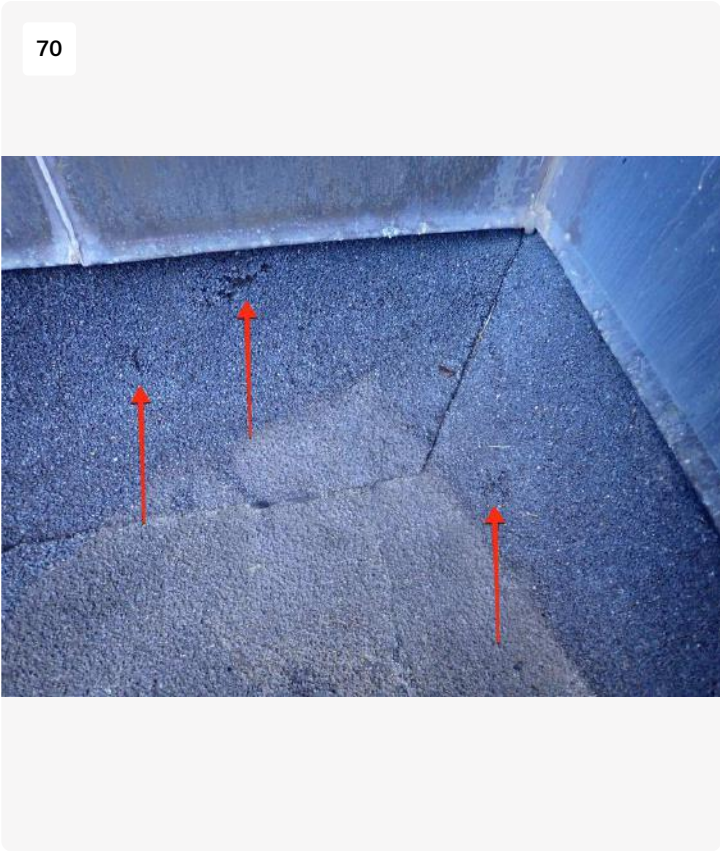
Damages to mod-bit from fallen tiles
