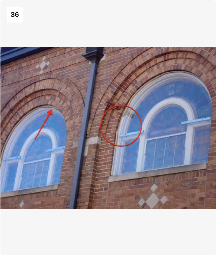
Damaged, missing window seal
