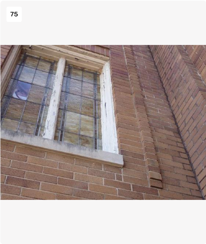
Damages to painted window frames due to high winds
