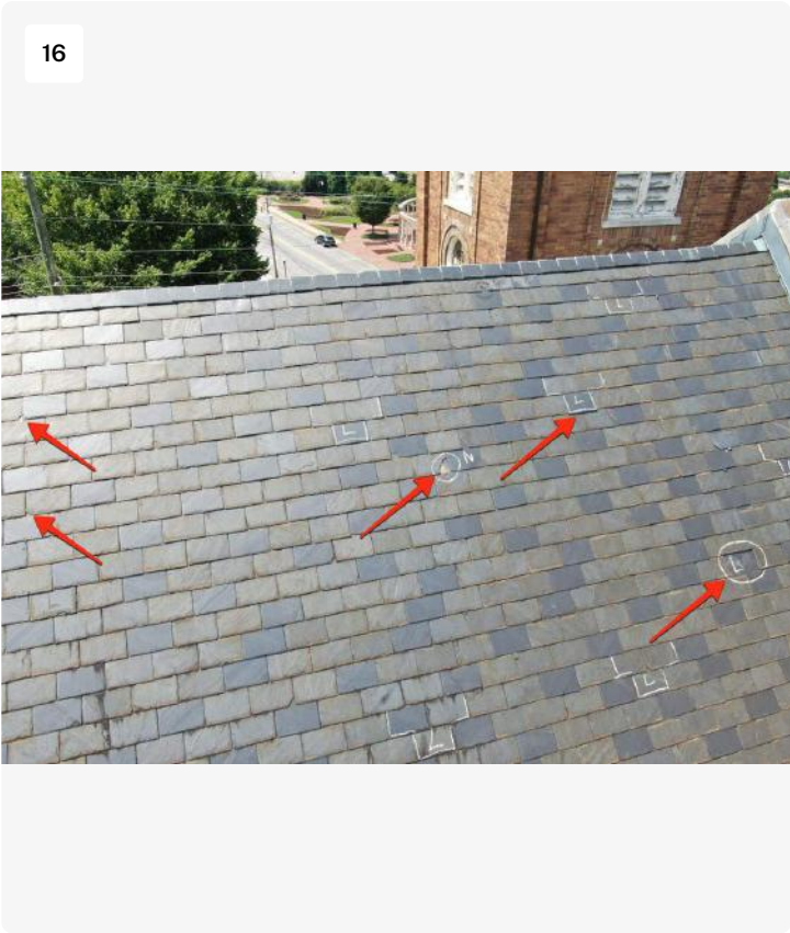
Cracked and displaced tiles
