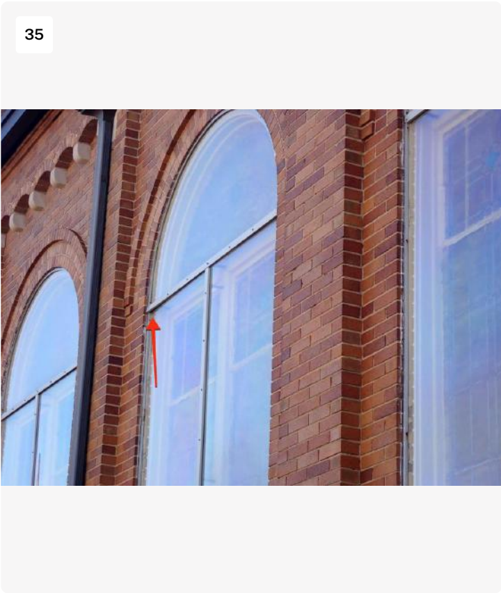
Displaced window frame
