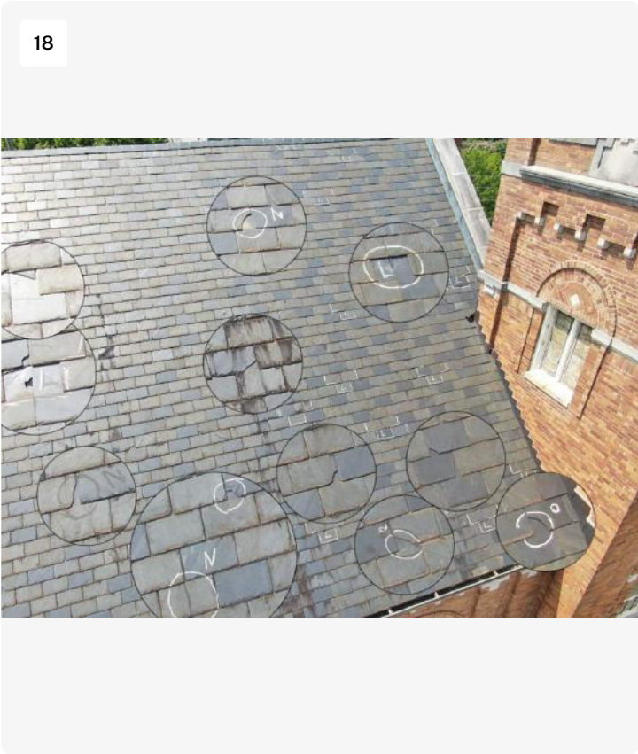
Missing, cracked and displaced tiles
