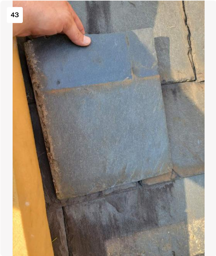
Displaced slate tile
