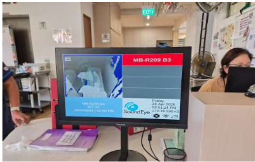
Monitors at nurse station
