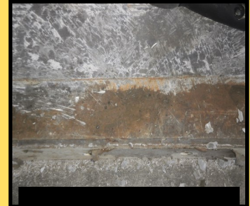
BX-543 10 Rust evident
