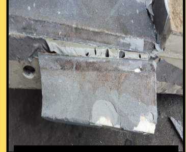
BX-543 02 Rust evident
