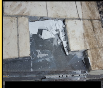
BX-543 01 Evidence of minimal tile adhesive used
