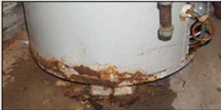
WATER HEATER/AC LEAKS
