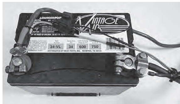
Completed Installation Shown
