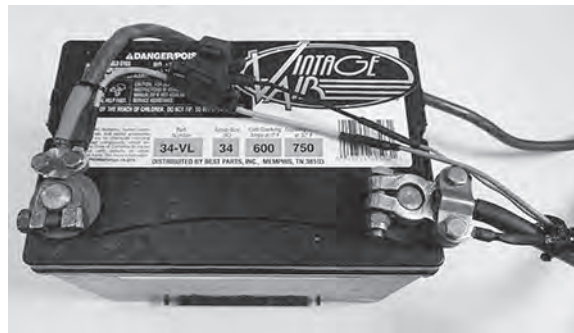
Completed Installation Shown
