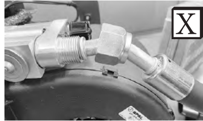
Improperly Seated O-ring Land
