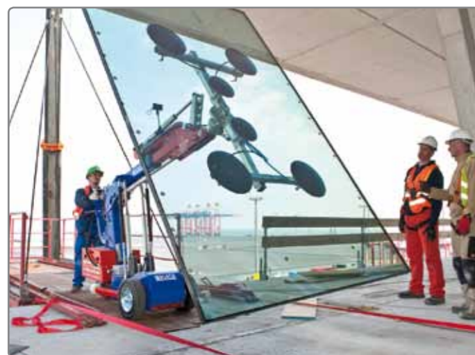
Construction site Jade Weser Port in Wilhelmshafen, Germany: the KS Robot glazes the facades with glass plates, approx. 500 kg.
