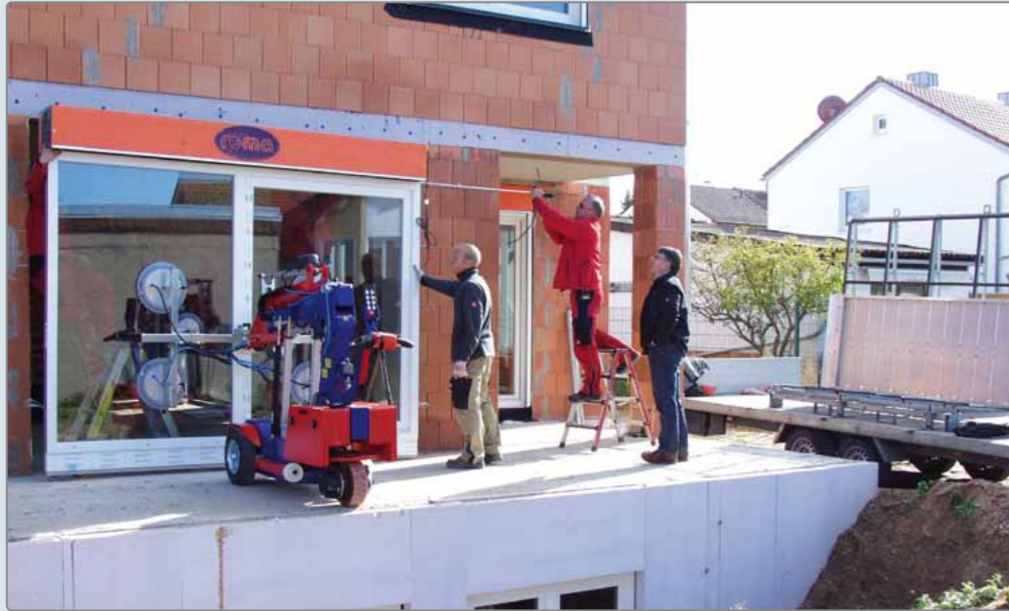
KS Robot 550 during installation of a lifting sliding door, company Busch, Wahlheim, Germany.
