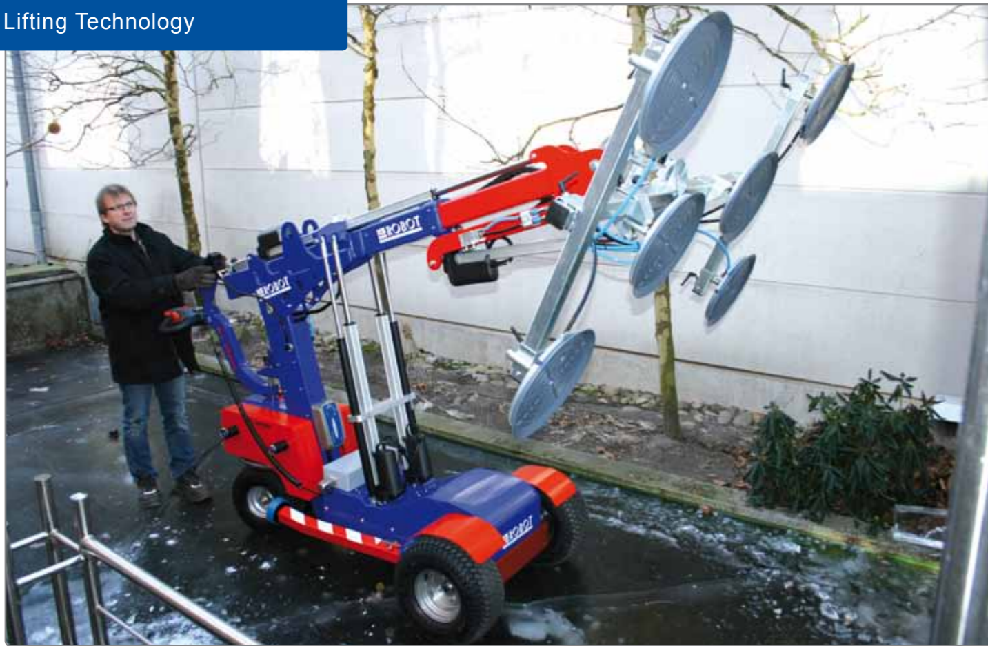
KS Robot 600 Offroad at an endurance test – even on ice the KS Robot scores. A frozen pond is the only possible access to make glass repairs in the roof glazing.
