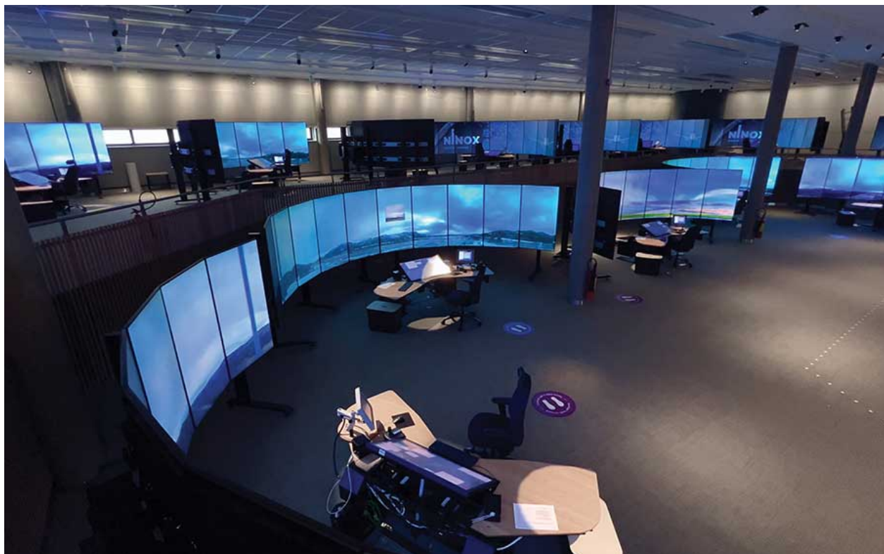
The centralized Indra Systems control center in Bodø, Norway currently is serving eleven airports, some of them hundreds of miles away. Eventually this one center will provide ATC services to all fifty airports in Norway, far less expensively and more efficiently than having fifty lightly-used towers scattered around the Arctic Circle.
