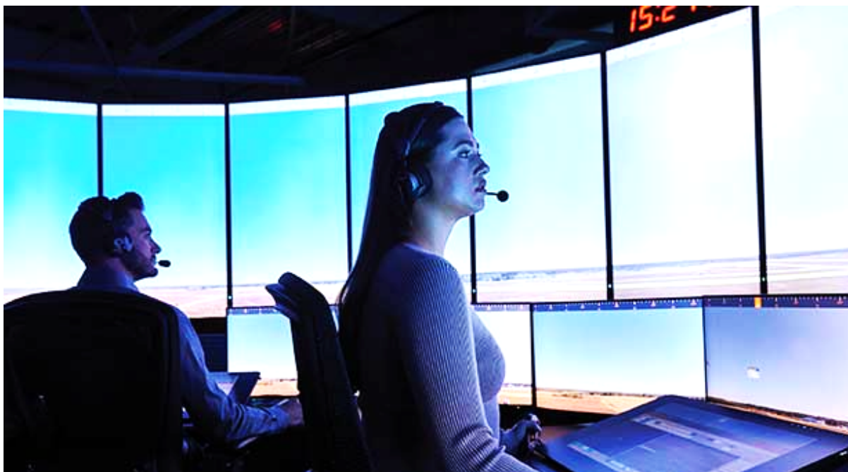
This is the Frequentis system installed at the FAA's Atlantic City Research Center, incorporating all the improvements Frequentis has developed in their first three prototype installations. This system is configured for the biggest and busiest airports, and could be simplified for deployment at less demanding airports. With luck, the FAA could finish testing and certify the system before year's end.
