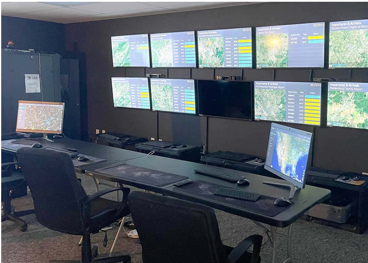
Photo 2: While so much in the “virtual” world is smoke and mirrors, VirTower is the real deal. It is a complete and operational company with two control centers (shown), trucks and installers, and a small army of software experts. This means they have the resources to accommodate new customers, fix problems, and develop new capabilities simultaneously.
