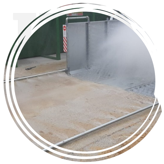
Inground Washing Lane
