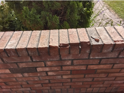
Some cracked brick at entrance
