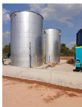
Lime Reactor Tanks
