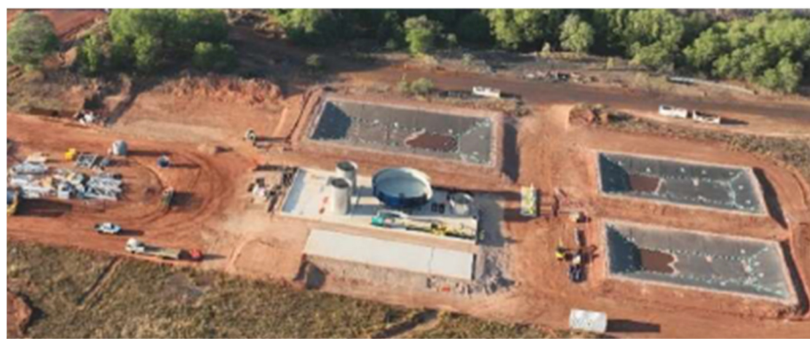
Aerial shot of the Ground Water Treatment plant
