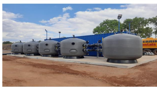
Operational Water Treatment Plant
