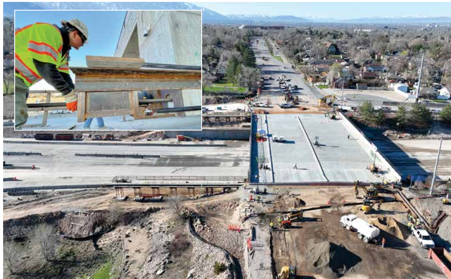
Action was fast and furious during the I-80/1300 East bridge slide April 15, as crews had to clear rubble from the demolition of the old bridge to make way for the new five million-pound superstructure. A complex system slowly inched the bridge forward, aided by the use of liquid soap to mitigate friction. (aerial courtesy UDOT; others by B. Fullmer)
