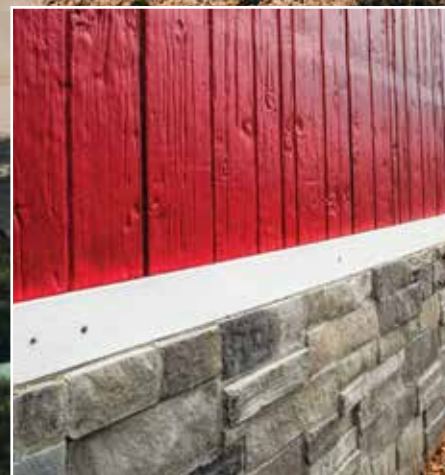
Sticky Bird in Farmington is a prime example of tilt-up versatility and the various exterior finishes that can be achieved. (courtesy AE Urbia)
