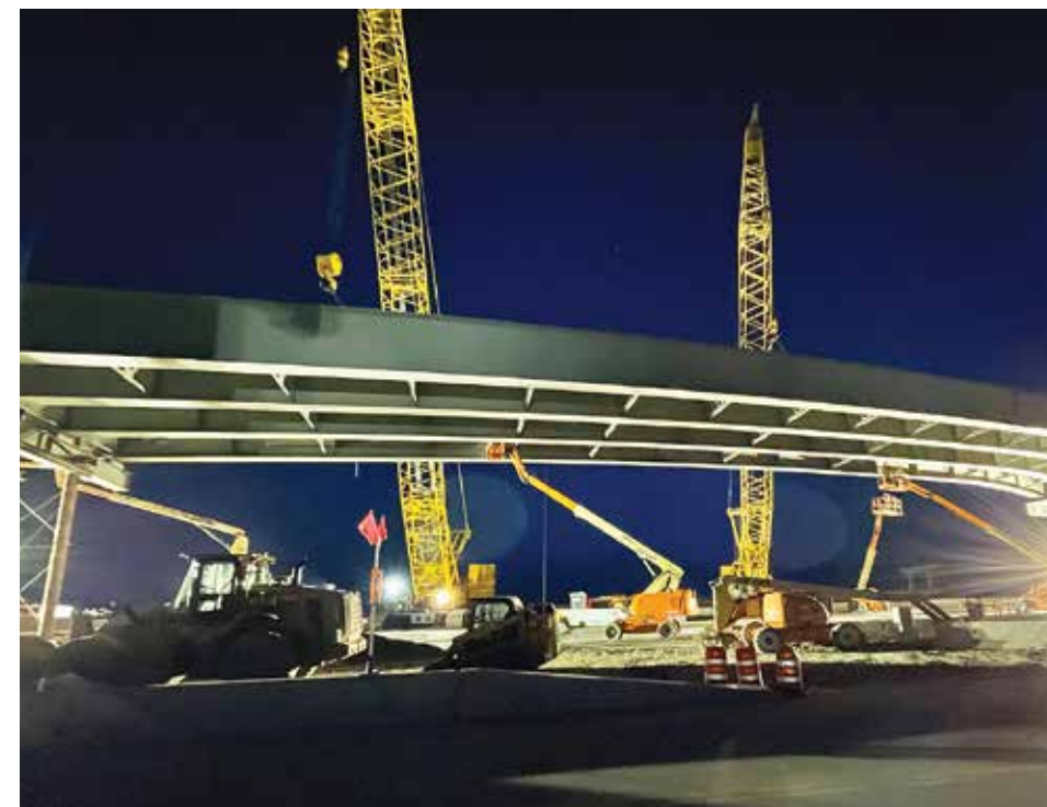
Crews from Farmington Bay Contractors place giant girders over I-15 April 16 as part of the bridge construction on the 16-mile long, four-lane, $800 million West Davis project.
