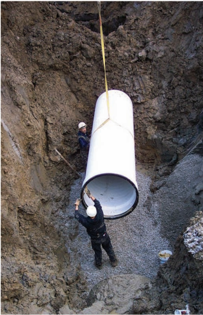
Bedding was critical to pipe placement. The triple gasket can be seen on this pipe segment.
