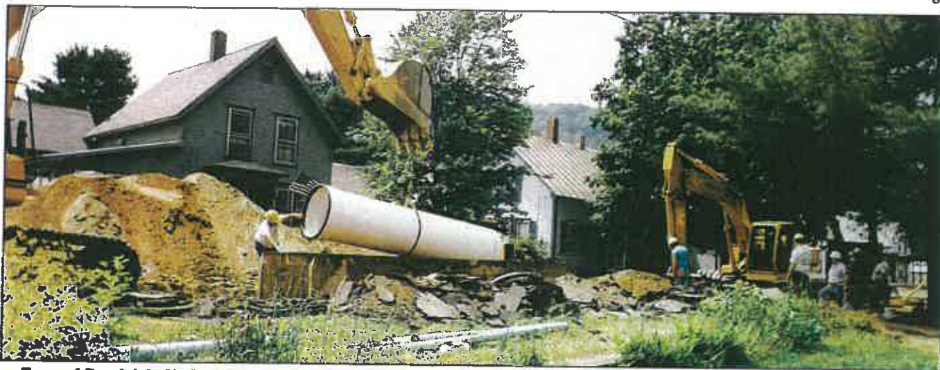
Town of Randolph, VT installs new stormwater system in response to combined sewer overflow (CSO) control policy.
