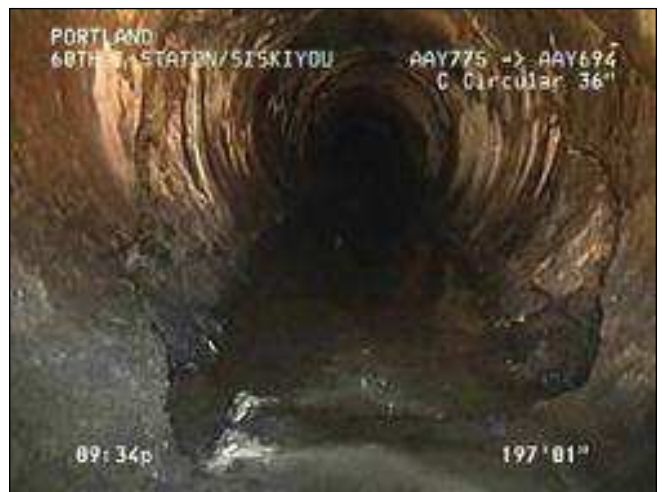
Existing deteriorated 36-inch sewer pipe
