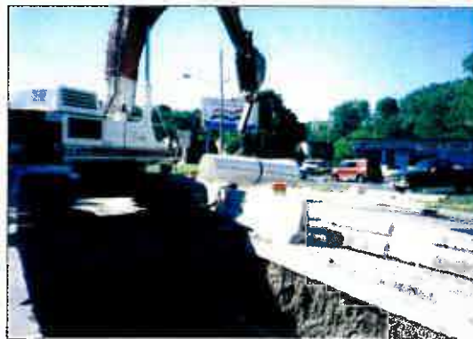
Marra Construction crews lower a 15-ft section of Lamson Vylon slipliner into the insertion pit.
