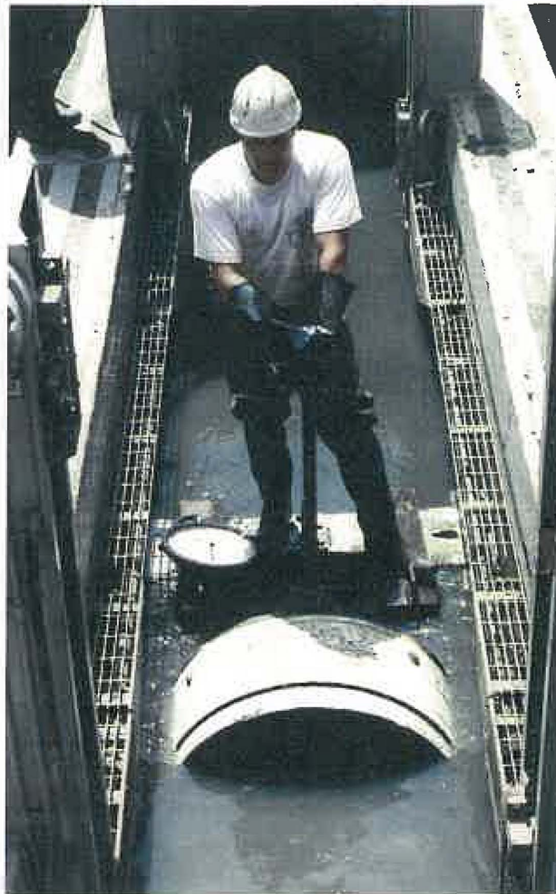
A crew member follows a short coupling section as it moves to join the pipe string.
