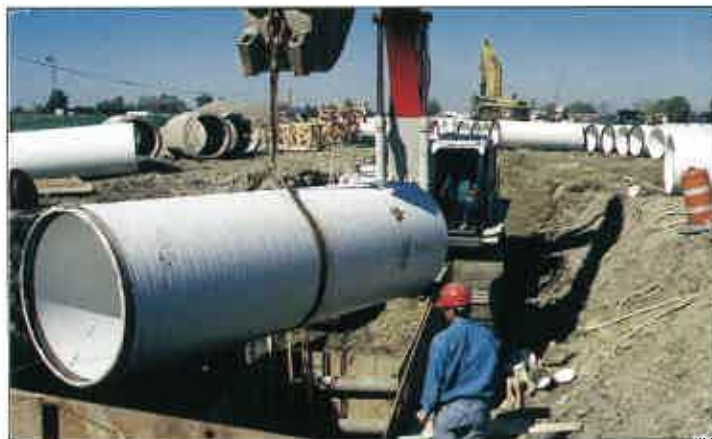
A section of pipe is lowered into an insertion pit. Pits were excavated at designated points along the pipeline and the host pipe was cut at the springline to allow for insertion of the slipliner.
