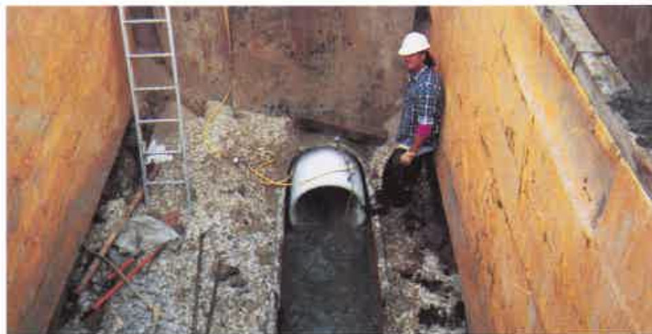
The old pipe is broken away in an entry pit so the liner can be slid into place.
