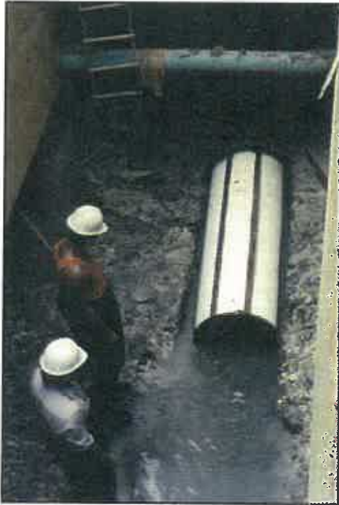
Boyer workmen watch as a mandrel begins a test run through the cleaned sewer.
