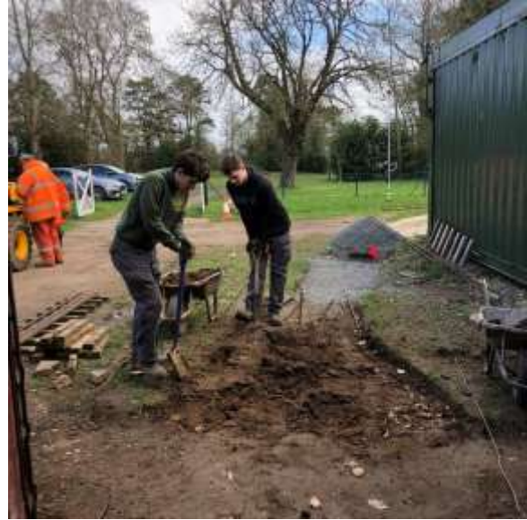
The lads were busy digging more soil out for us to suit the permanent fixed rails.
