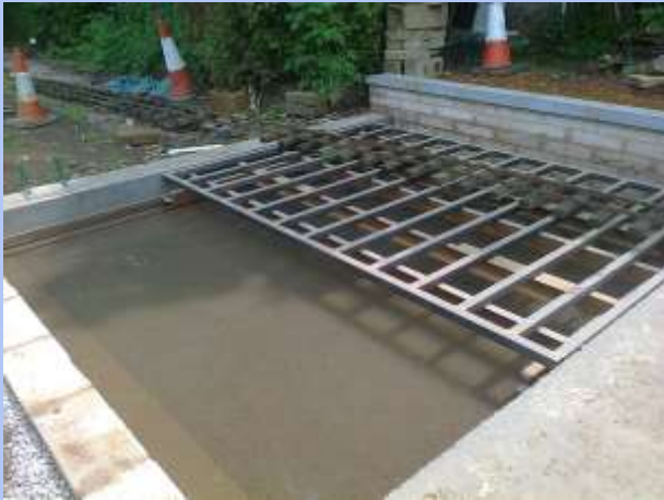
We experienced our first flooding of the new traverser pit following a heavy downpour.
