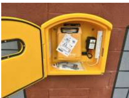
The defibrillator unit inside the cabinet.
