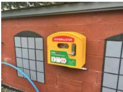
The new cabinet looking smart. Please help to keep the area clear so that it can be accessed easily if needed.
