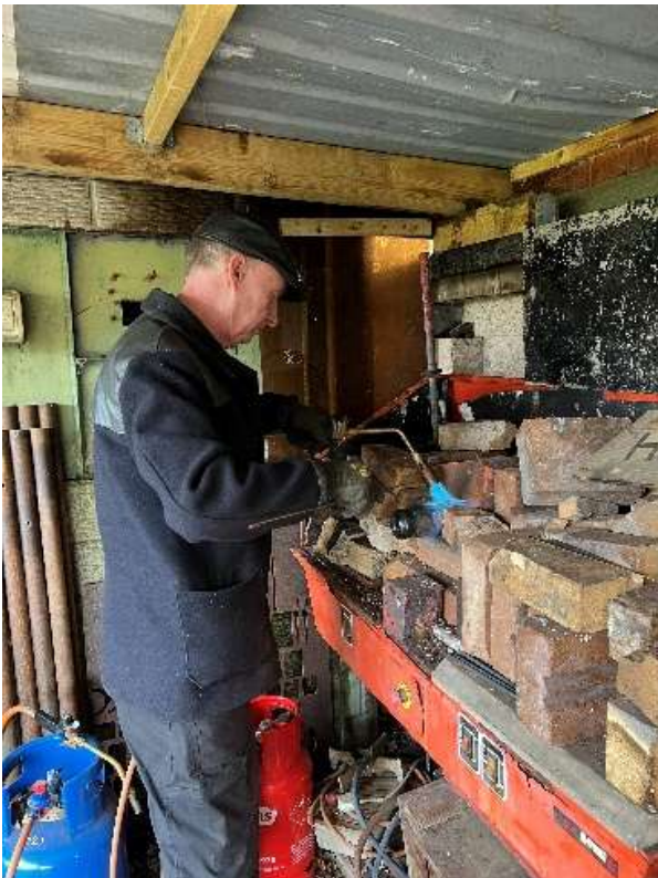
George working on a repair to part of the vacuum brake system
