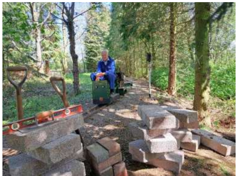
John Powell delivering concrete for the footings by rail on 22nd April.
