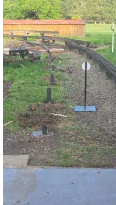
The post bases were concreted in the ground ready for the track support posts.
