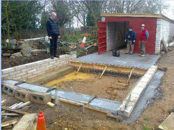
Walling going in around the traverser pit overseen by Aubyn, Tony and Geoff.
