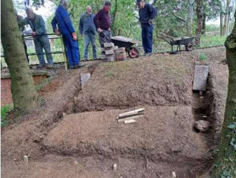
The Ballast Washing Plant footings ready for concrete – Pete, John & John Geoff and Bernard in attendance.
