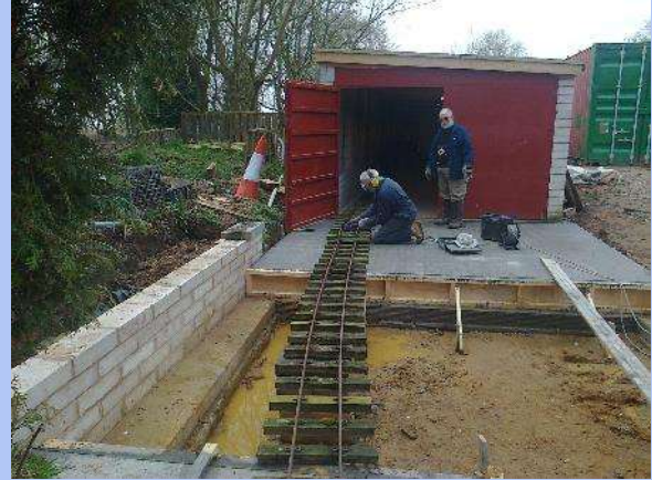
Temporary track going in so carriages can move in and out over the pit.
