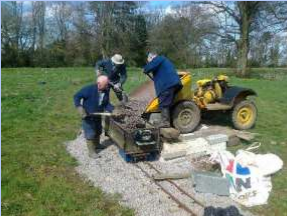
Loading the ballast truck from the Dumper - at this point we were working on the inner loop of the extension.
