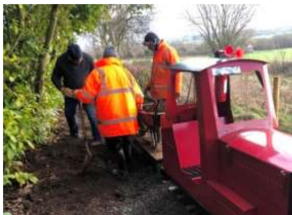
Loading up the excess soil using the flat waggon and two wheelbarrows pulled by 'Rufus'
