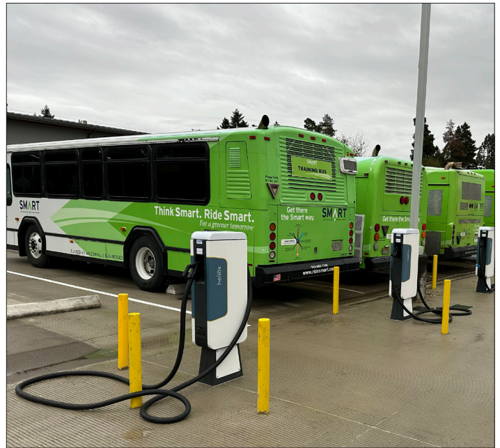
The Wilsonville SMART facilities expansion equipped the site charging facilities for buses and public works vehicles.
