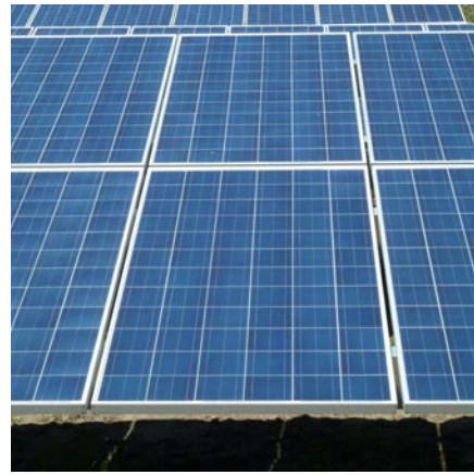
River Falls Municipal Utilities solar array
