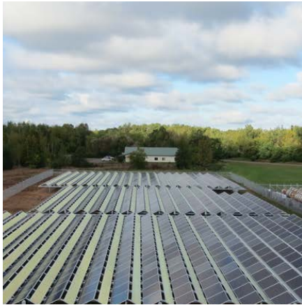
Bayfield Electric solar garden
