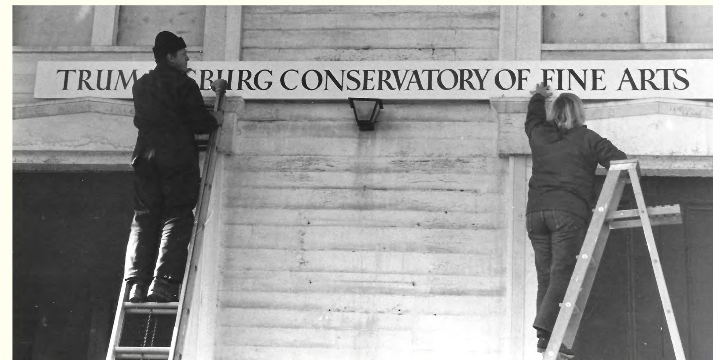
The new TCFA sign being installed above the front doors. Photo courtesy of The Ulysses Historical Society
