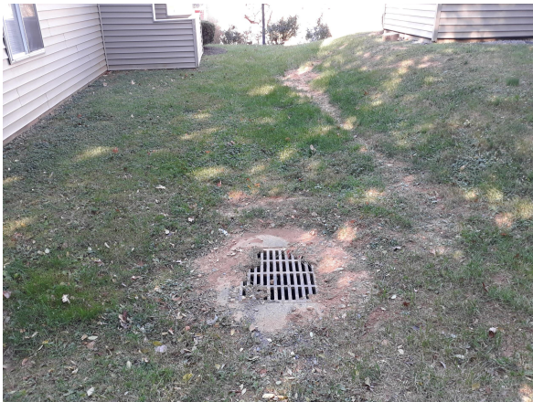
Debris in storm drain
