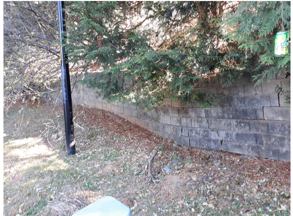
Damaged retaining wall
