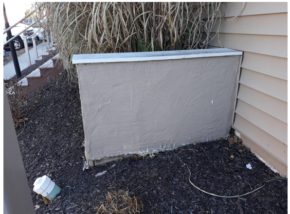
Damaged stucco finish
