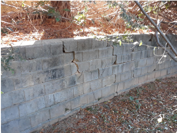
Damaged retaining wall
