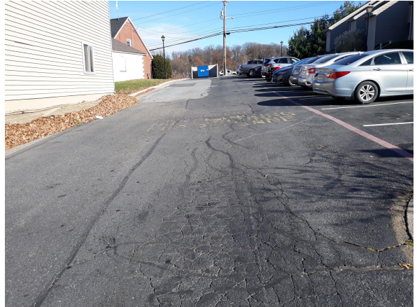
Asphalt surface worn
