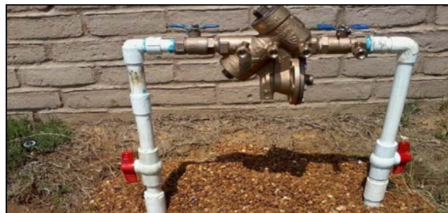
Example Installation of Irrigation Backflow Preventer
