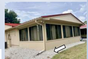
Erosion control - Parish Office
