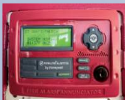
Fire Alarm system
