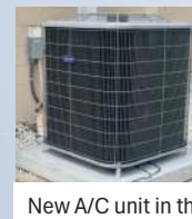
New A/C unit in the Education Bldg.
