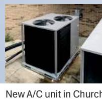
New A/C unit in Church Unit 1
