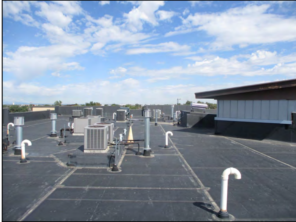
35: Roof profile and A/C equipment
