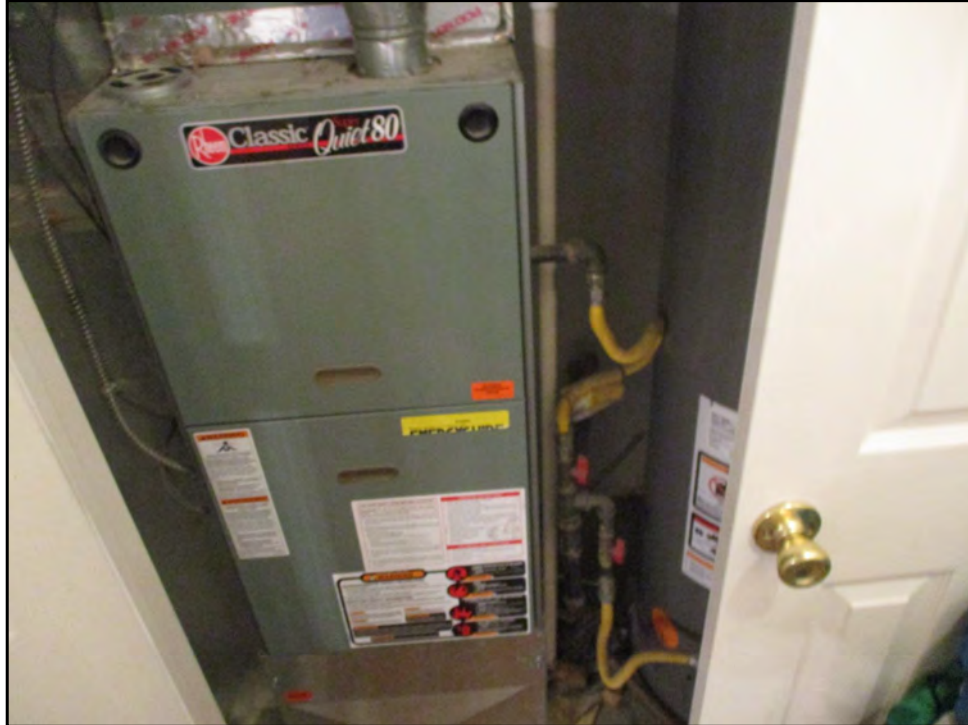
133: Replace unit and common area furnaces (Immediate Repair)
