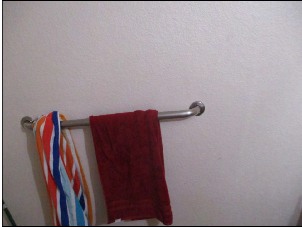
169: Non-compliant grab bars at HC unit toilets (Immediate Repair)
