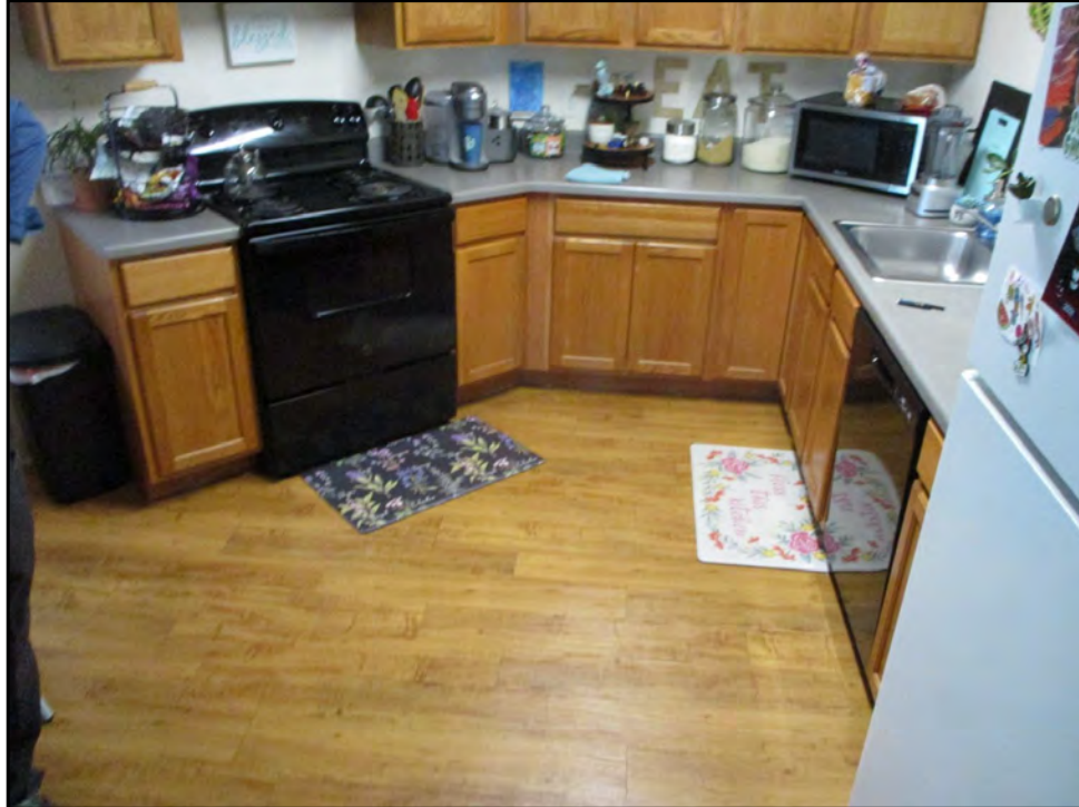
89: Interior dwelling unit. 3 Bed/ 2 Bath Type F unit without 48-inches at the base of the U (Immediate Repair).
