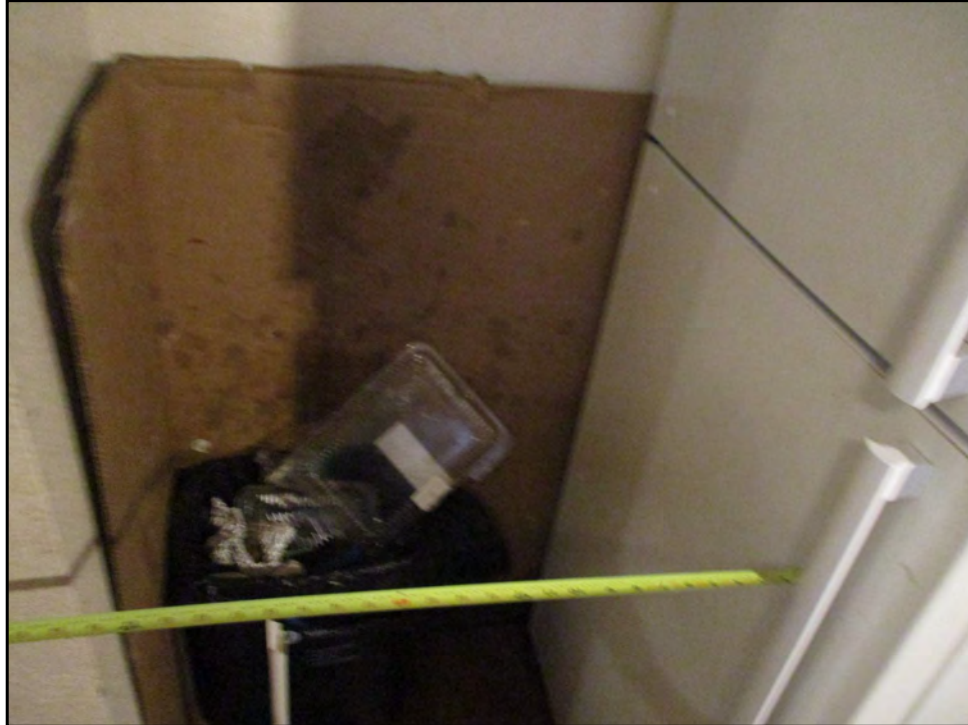
167: Missing compliant approach to refrigerator within Type C units (Immediate Repair)
