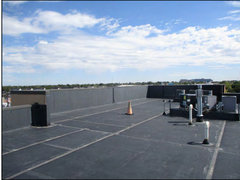
129: Replace roofing membrane (Immediate Repair)
