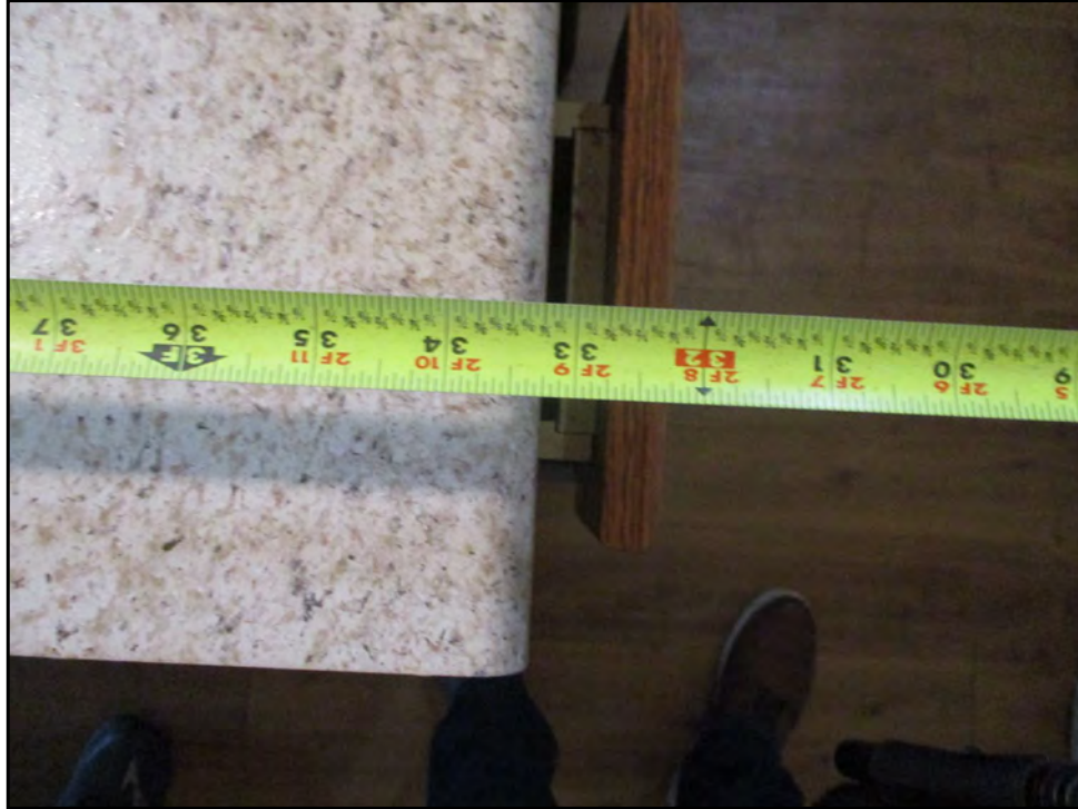
159: Missing compliant maneuvering space within galley kitchens in Type J floorplans (Immediate Repair)
