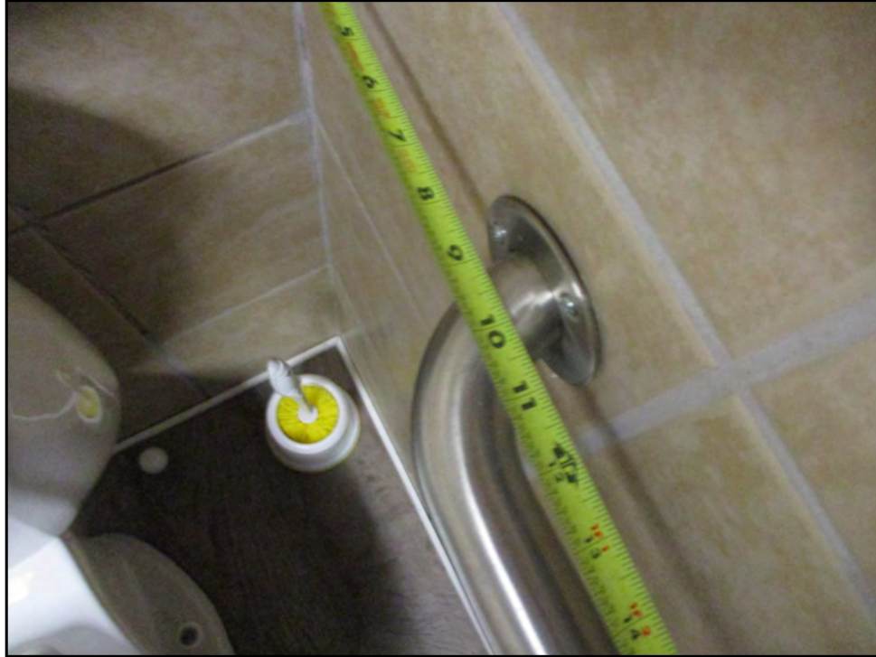
151: Non-compliant toilet grab bar at common restroom (Immediate Repair)
