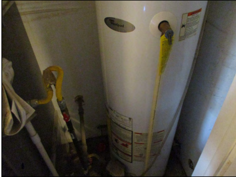
131: Replace dwelling unit water heaters (Immediate Repair)
