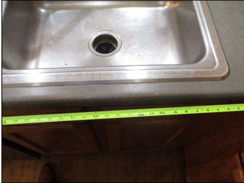
157: Missing 30x48-inch parallel approach to kitchen sinks at unit Type D (Immediate Repair)
