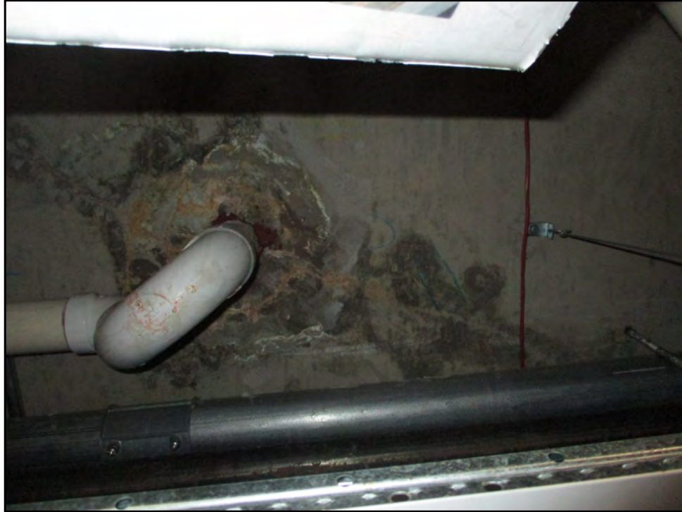
119: Water leaking around floor drains (Immediate Repair)
