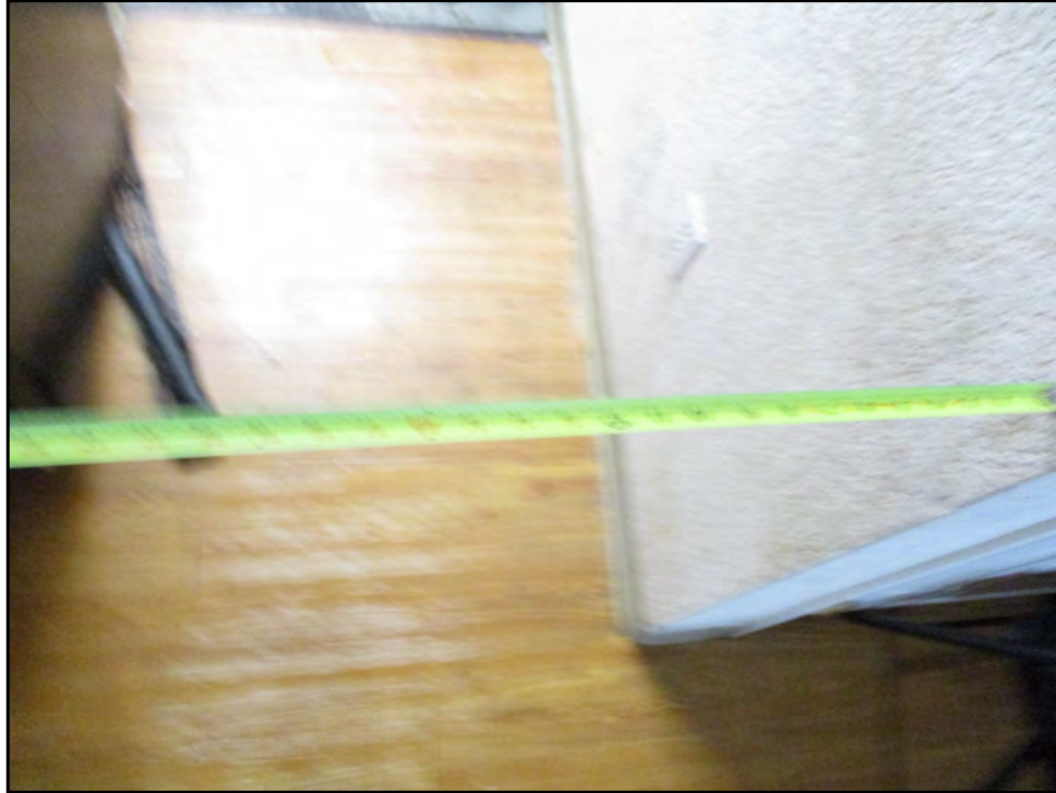
165: Missing compliant maneuvering space within galley kitchens in Type K units (Immediate Repair)
