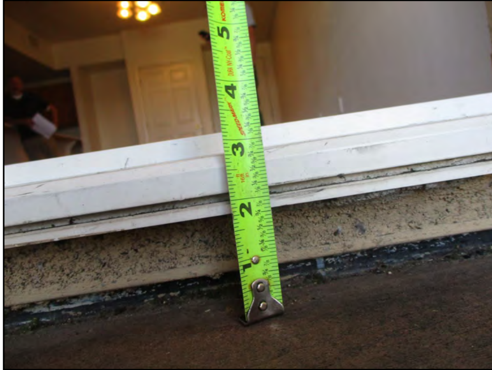
143: Reconfigure thresholds at patio sliding glass doors (Immediate Repair)
