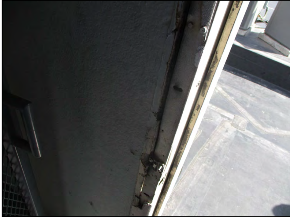
127: Repair damaged roof access door and frame (Immediate Repair)
