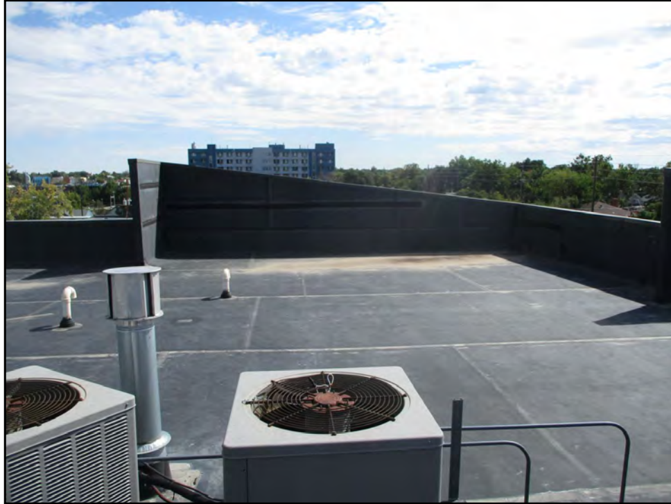
37: Roof profile and A/C equipment
