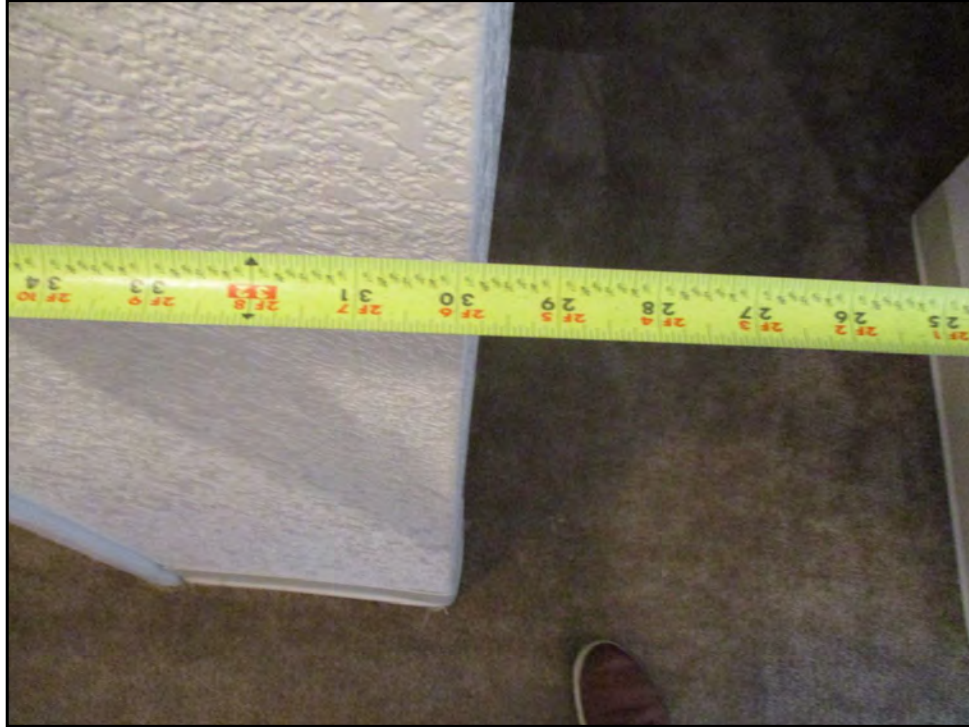
155: Master closet in Type J less than 32-inch wide openings (Immediate Repair)
