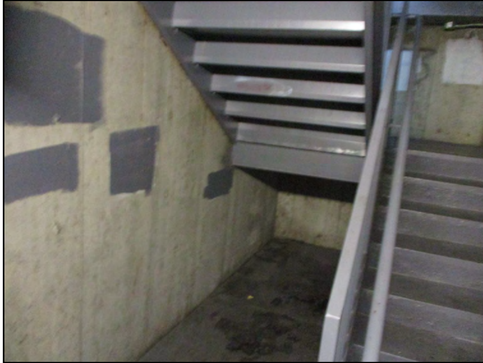
121: Missing cane detection beneath staircase assembly (Immediate Repair)
