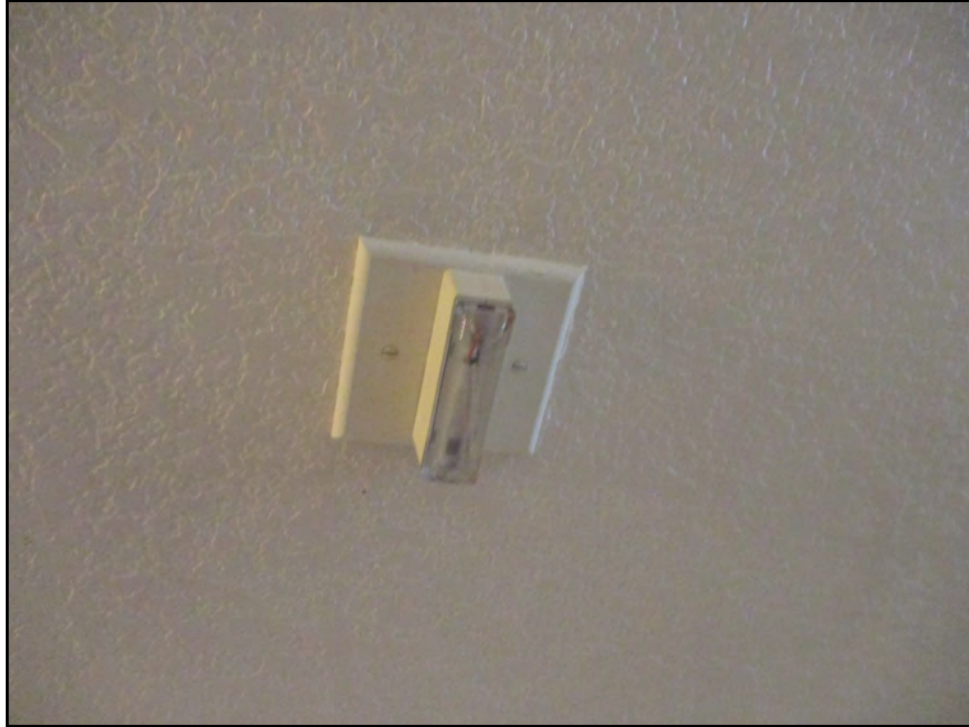
149: Install A/V alarm in non-HC dwelling unit (Immediate Repair)
