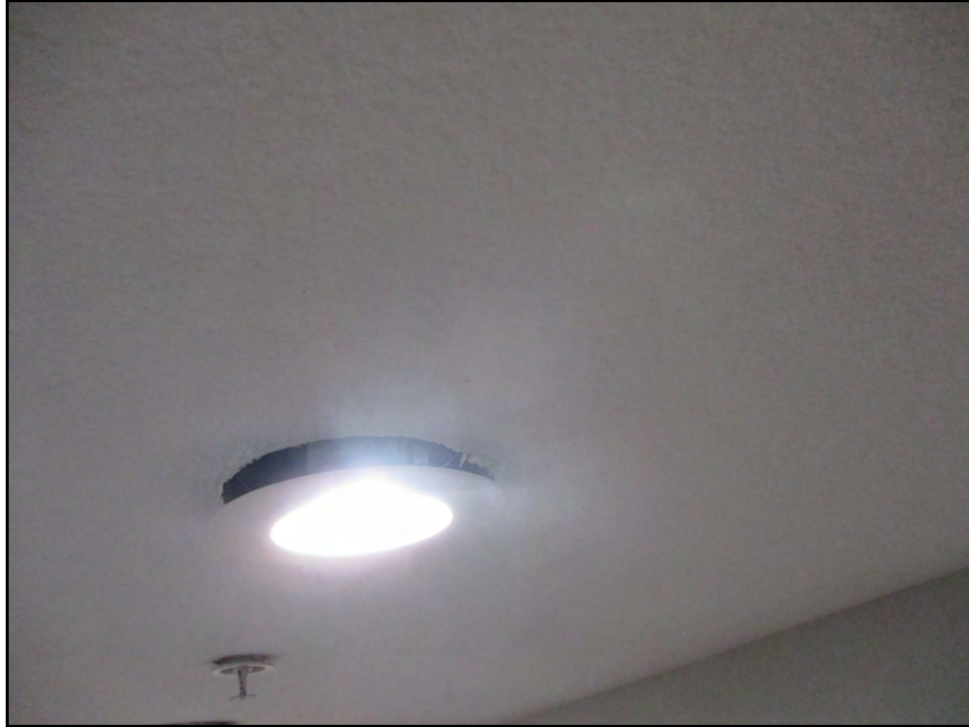
125: Repair common area lighting (Immediate Repair)
