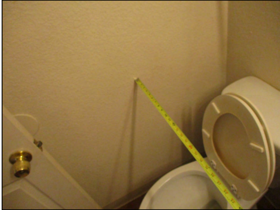
171: Less than 33-inches between wall and vanity at toilet in select floorplan types (Immediate Repair)
