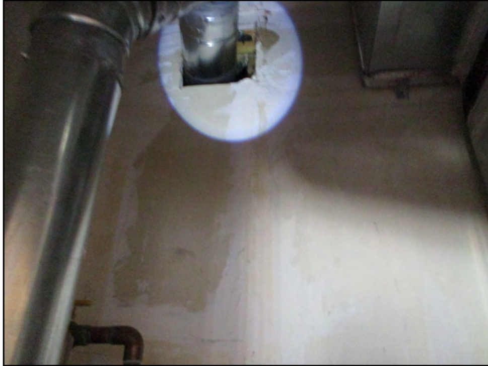
173: Unsealed thru-wall penetrations at unit mechanical closets (Immediate Repair)
