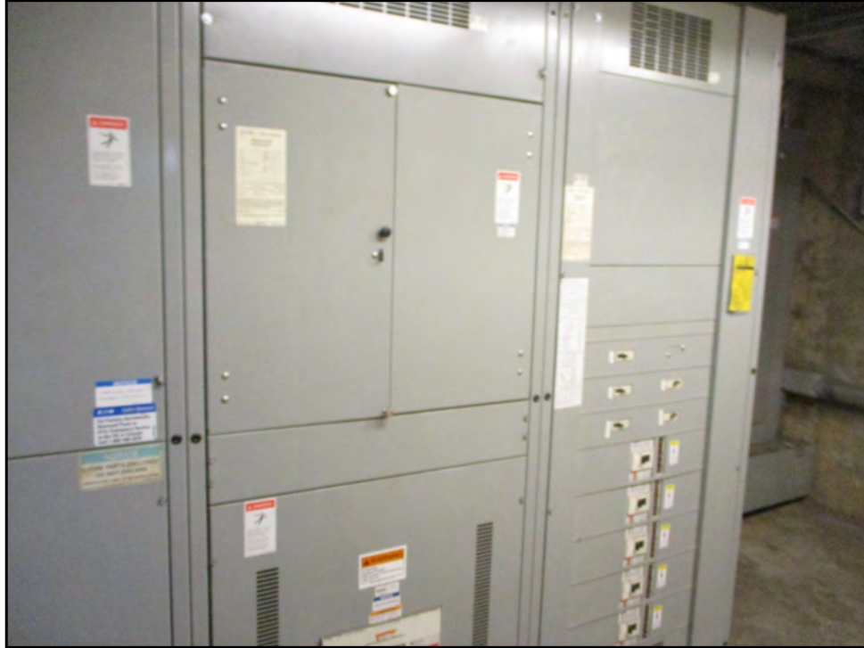
45: Main electrical equipment
