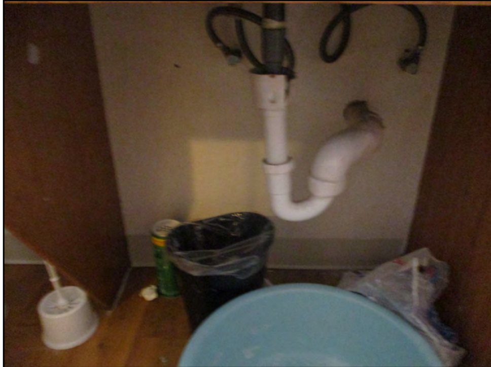
163: Missing scald and abrasion protection at kitchen and bathrooms sinks in HC units (Immediate Repair)
