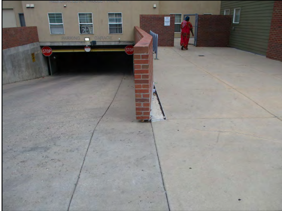
123: Repair damaged wall at parking garage (Immediate Repair)
