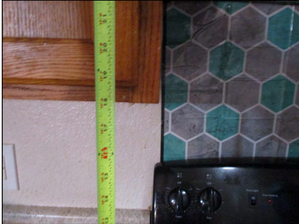
161: No lowered shelving in HC unit (Immediate Repair)
