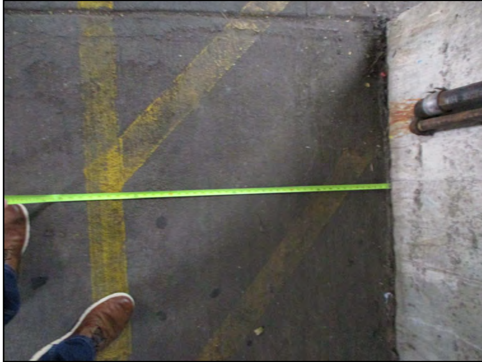
141: Repair non-compliant access aisle at HC parking spaces (Immediate Repair)
