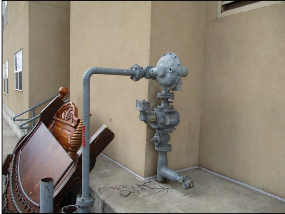
31: Main gas supply
