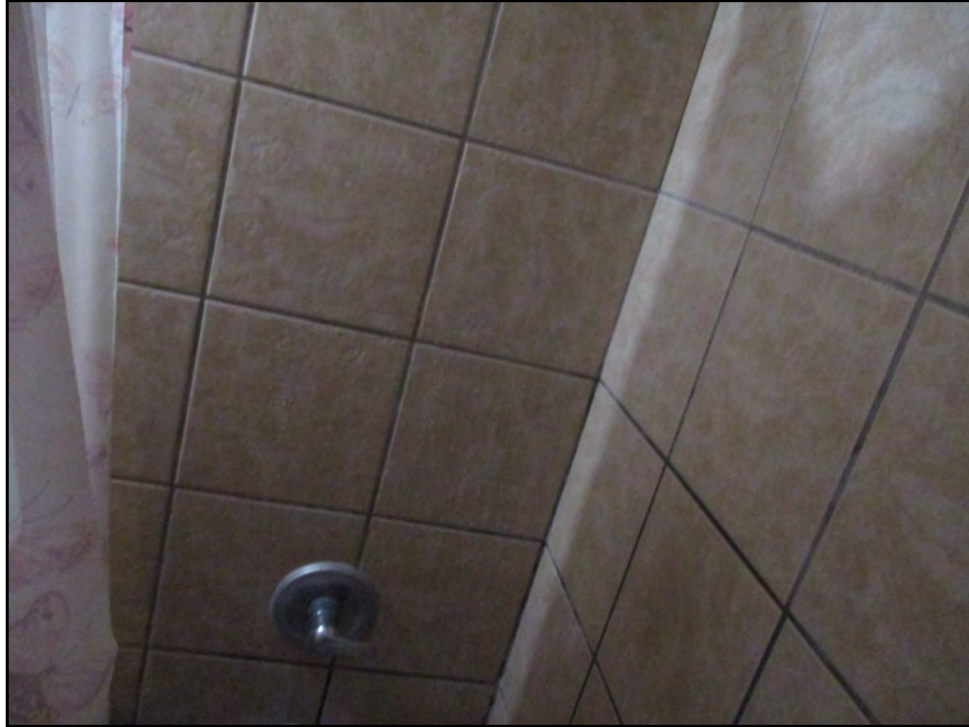
147: Missing shower spray unit at HC units (Immediate Repair)
