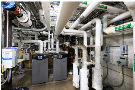
Piping in the Boiler Room for HVAC
