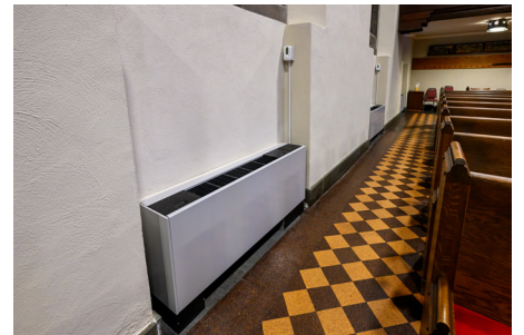
New fan coil units throughout the sanctuary
