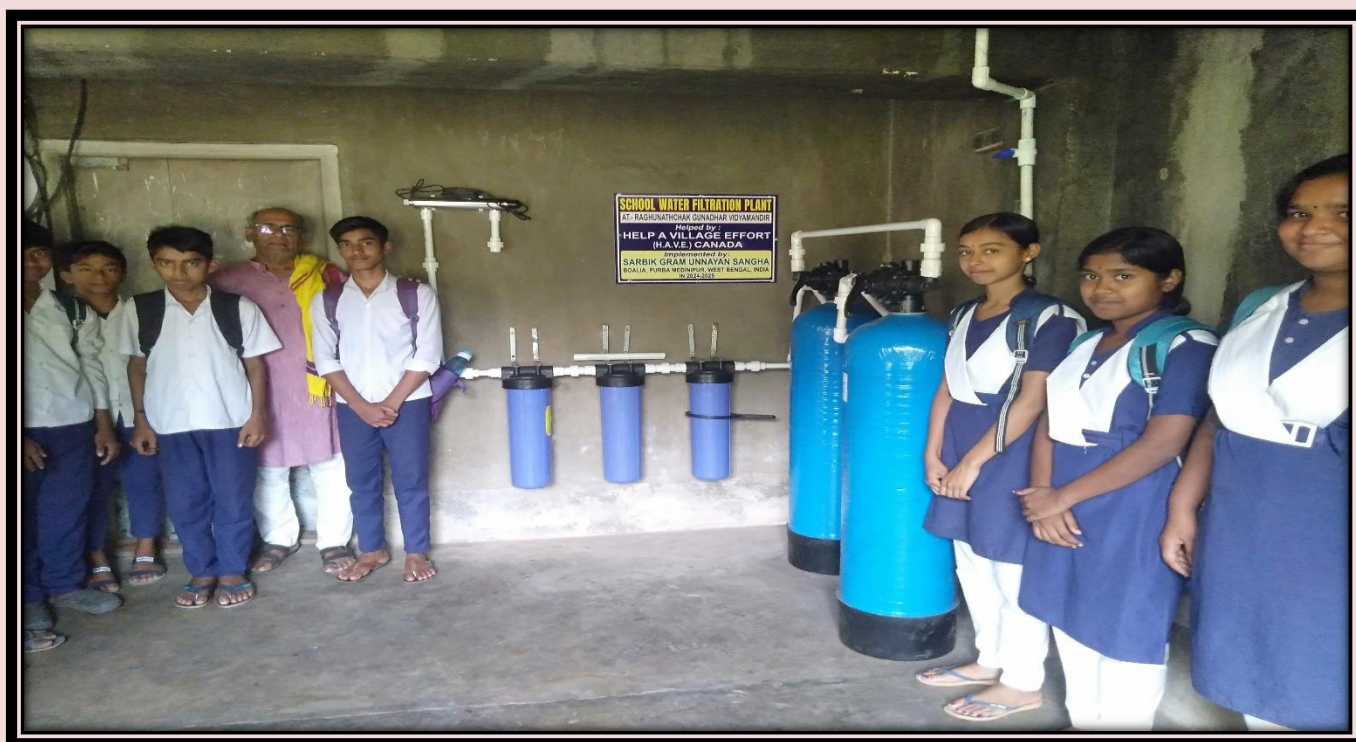
Raghunathchak Gunadhar Vidyamandir Water Filtration Plant.
