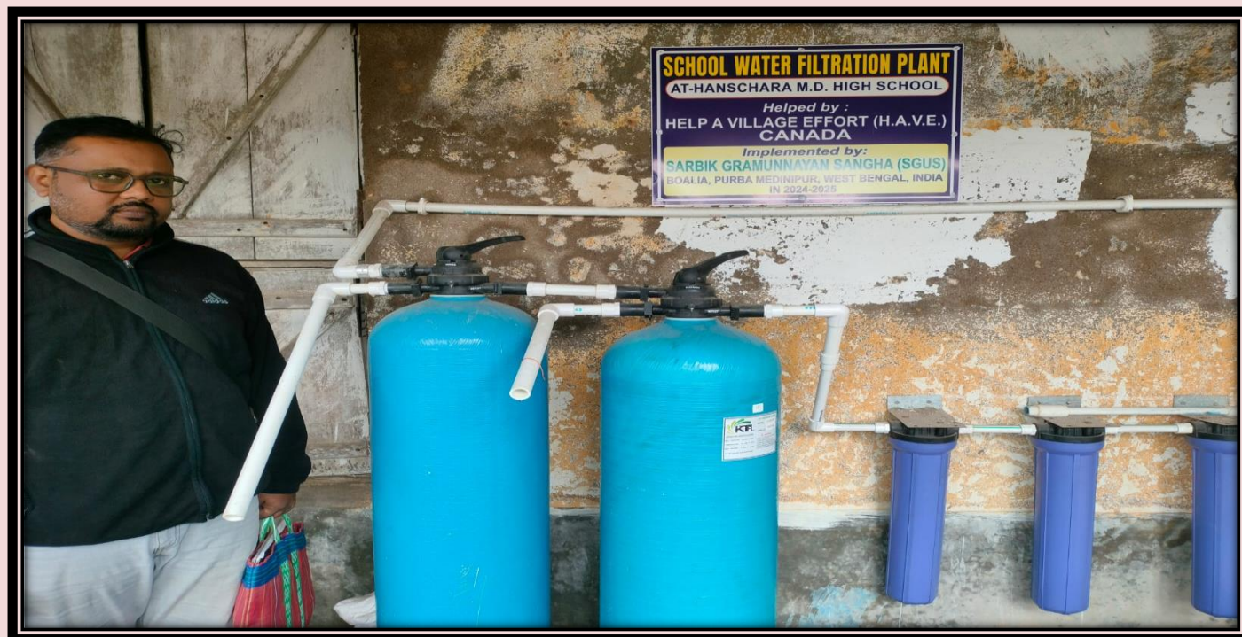
Hanschara M.D. High School Water Filtration Plant
